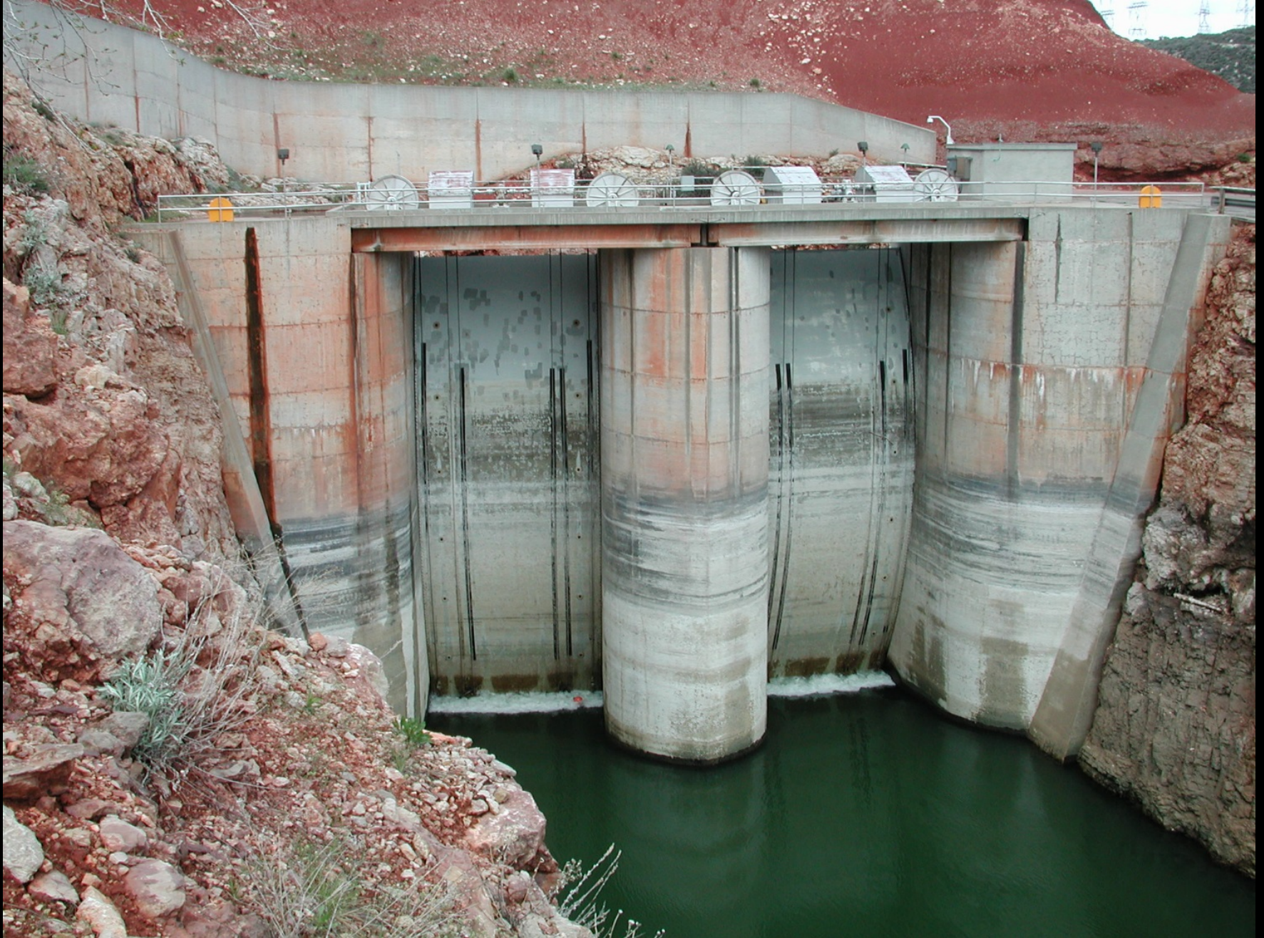
April 27: Elevation 3606.7': 2' Head on Gates
