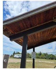
Fish Cleaning Station
