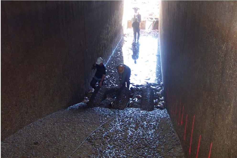
Choke Canyon Dam River Outlet Works, Nueces River Project, Choke Canyon Dam, Texas
