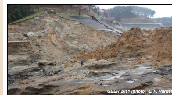
Figure 10: View of Breach in Fujinuma Main Dam from Left Abutment Looking Upstream (N37.3021°, E140.1952°, April 23, 2011)
