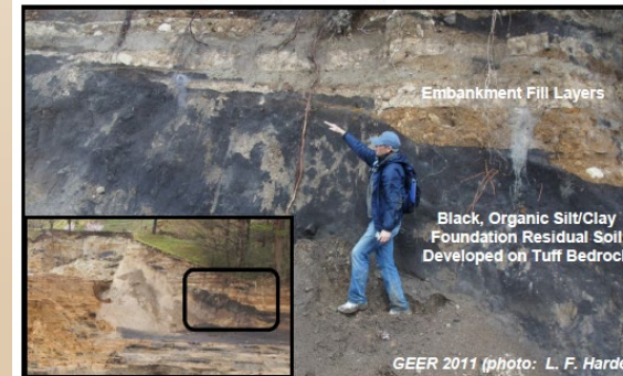
Figure 14: View of Fujinuma Dam Embankment Fill Layers On Top of Black Organic Foundation Residual Soil Exposed within Downstream Slope at Left Abutment (N37.3024°, E140.1951°, April 23, 2011)
