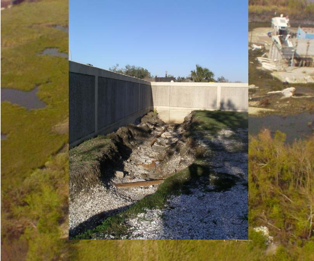
Figure E-8-5.—Overtopped Type II I-wall with damage but no failure.
