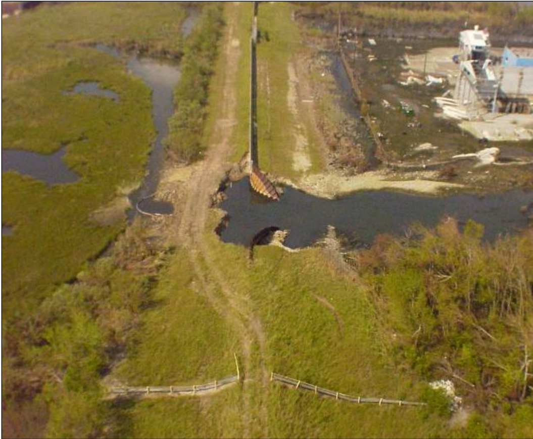
Figure E-8-4.—Failure of sheetpile I-wall due to overtopping.
