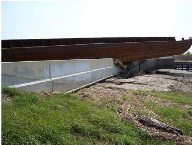
Figure E-8-8.—example damage from a barge impact during Hurricane Katrina.
