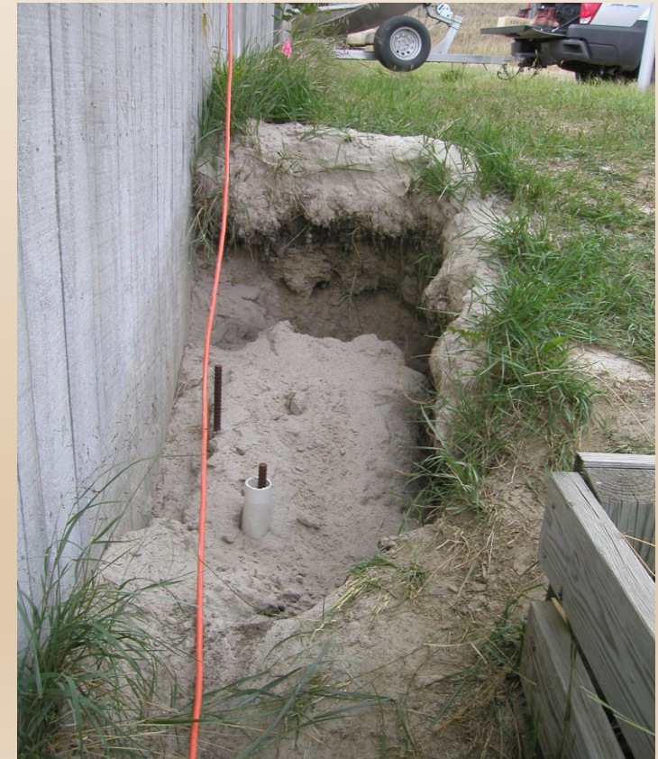
Photo 1 – Sinkhole on 9/27/2007 showing settlement of sand which was placed in hole in May 2007.
