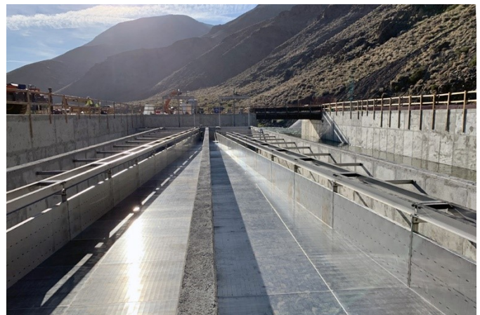
Nation's largest horizontal fish screen at Derby Dam
