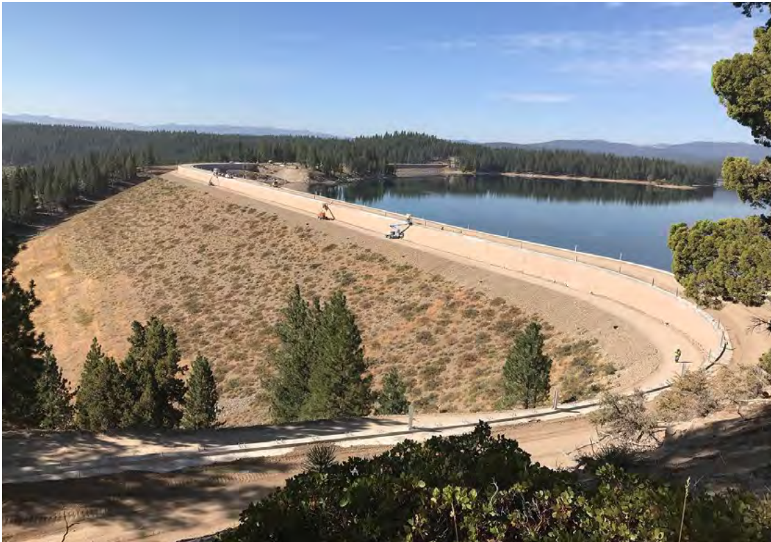
Figure 28. Downstream face of Stampede Dam, California, showing construction of the 11.5-foot-high crest raise.
