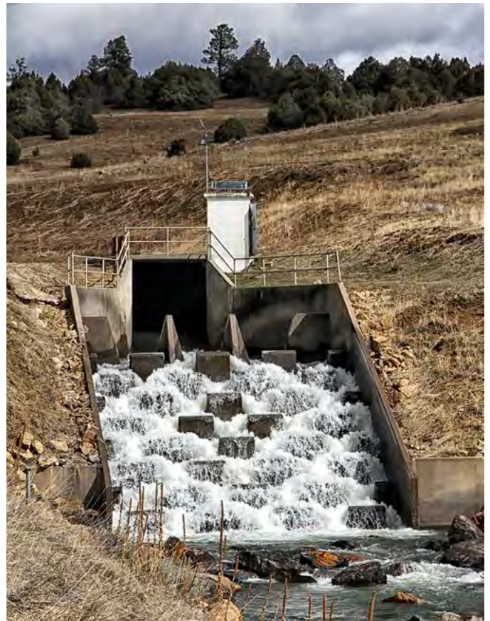
Figure 8. Azotea tunnel outlet near Chama, New Mexico releasing to the Rio Grande Basin the water diverted from the San Juan basin in Colorado as part of Reclamation’s San Juan-Chama Project.
