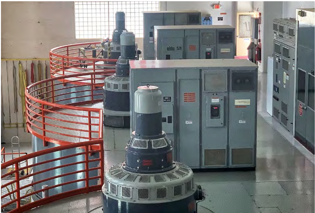
Figure 15. In New Mexico, Elephant Butte Dam generators operate only during irrigation releases for the Rio Grande Project, which are typically between April 1 st and September 15 th , but can occur for periods as short as 1 month.
