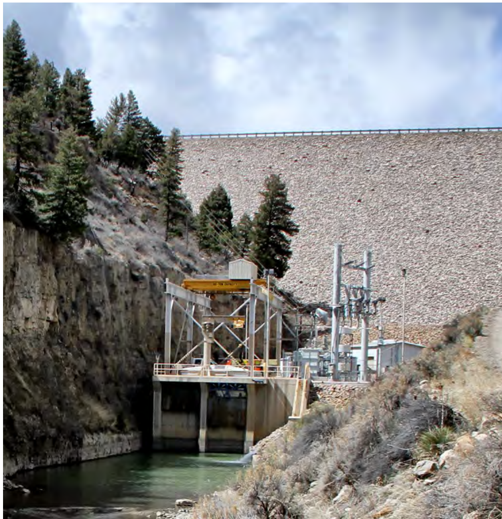
Figure 32. This hydroelectric powerplant below El Vado Dam is owned and operated by Los Alamos County, New Mexico.
