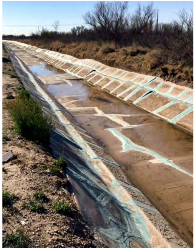
Figure 21. Carlsbad Irrigation District WaterSMART project to conserve water through reduction of seepage losses from an irrigation canal.
