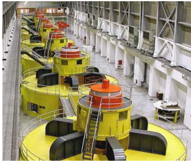
Hydropower generators at Glen Canyon Dam, Arizona.
