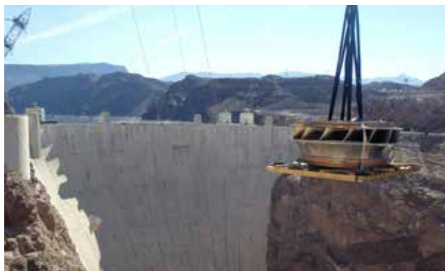
Delivery of a new wide-head turbine runner for Unit N-5 at Hoover Dam. The turbine arrived on a flatbed truck wrapped in a protective tarp and was flown in using an overhead crane.
