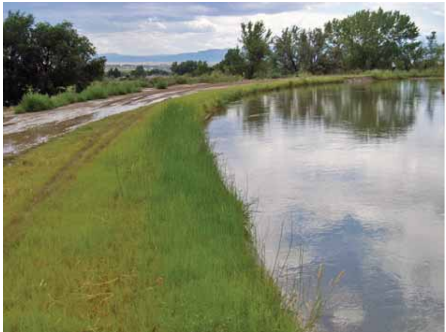
Water levels are impinging on the freeboard.
