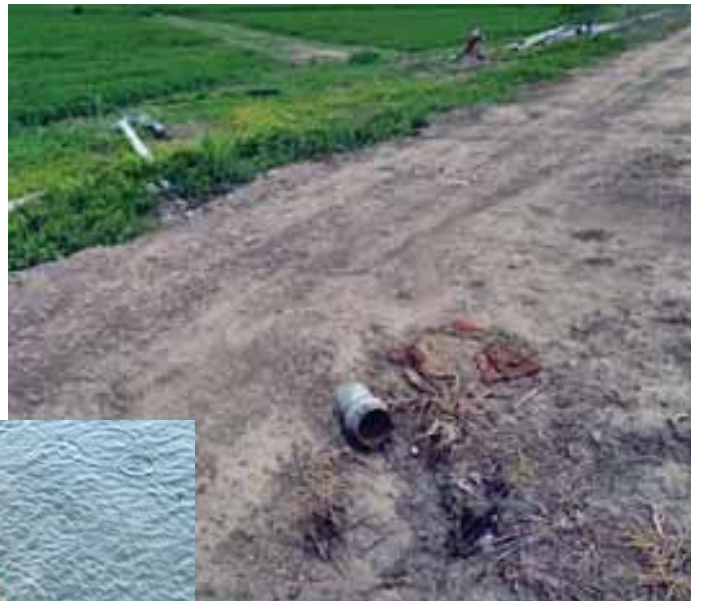
Unauthorized pipe (above).
