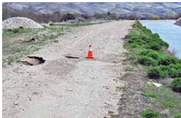
Try to determine the cause of the void and repair as quickly as possible.
