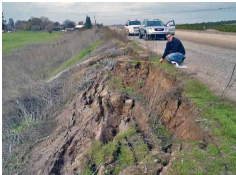
Sloughing of the outside slope of the canal embankment.
