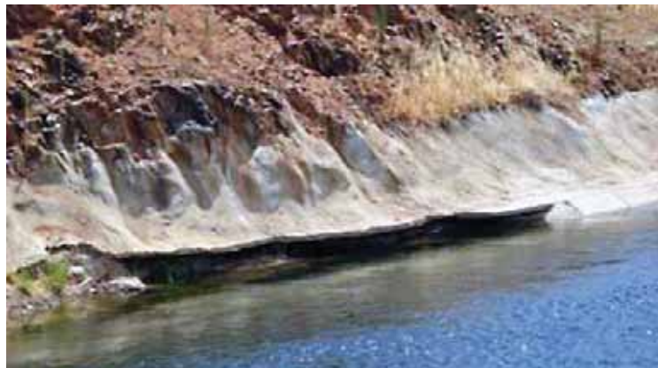
Erosion on left inner bank at cut section below shotcrete lining.
