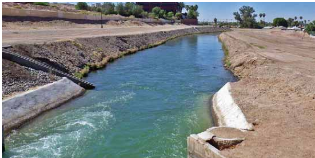
Downstream from the check gate structure. Notice the turbulence in the water extends past the length of the concrete transition, causing scour to the unprotected canal sidewalls.
