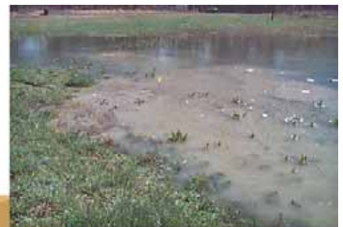
Cloudy seepage at the embankment toe is a sign of internal erosion.
