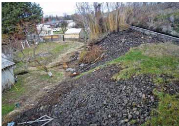
The backyard at the toe of this concrete canal flume embankment shelters trees and harbors seepage from the canal.
