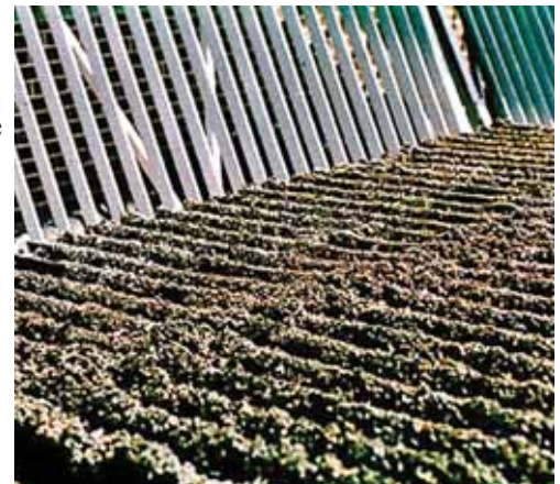
Quagga mussels on trashrack.
