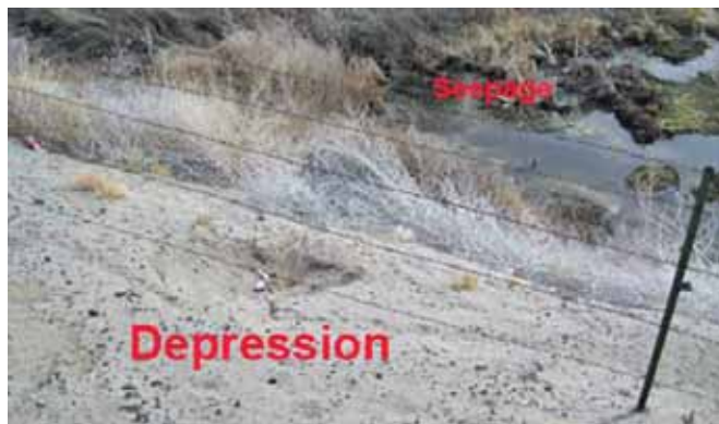
The depression on this embankment is just above a seepage area on the embankment toe.
