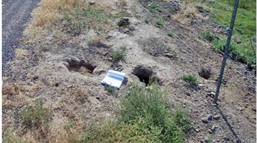
Rodent holes on the outside can pipe and cause erosion too.
