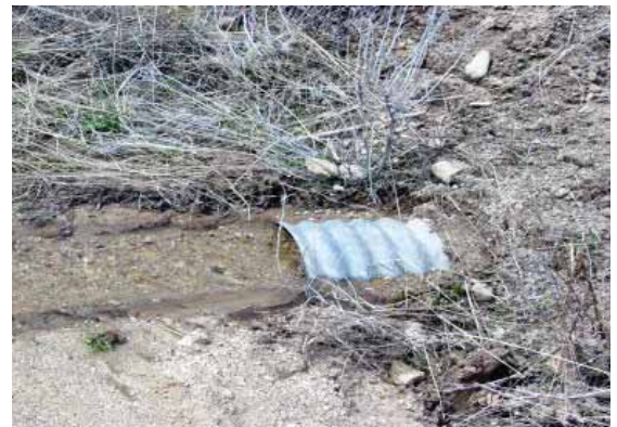
Plugged CMP culvert.
