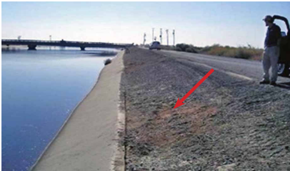
Water operations exceeded the top of the concrete lining, scouring the canal embankment.
