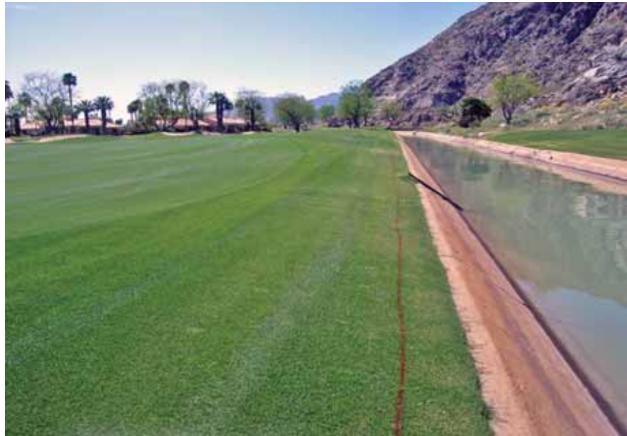
Golf course grading of this fairway removed the earthen freeboard.
