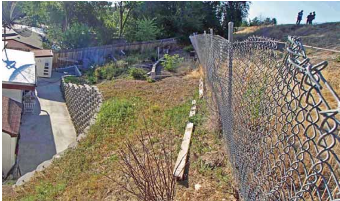
Because of this retaining wall, water only needs to seep through ten feet of embankment to inundate this property rather than through the wider original embankment.
