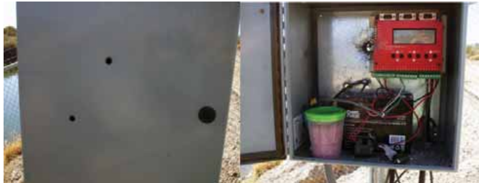
If there are bullet holes in the cover (left) and interior (right) of the equipment, inspect for damages.
