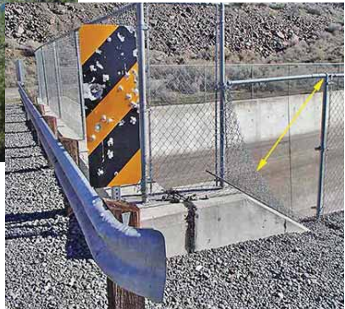
Shot-up sign and cut chain-link fence.
