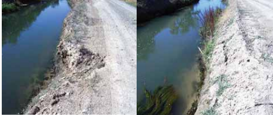
Erosion/ sloughing on the inside prism (left).
