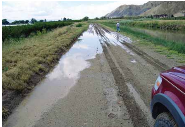
Poor road maintenance has resulted in a berm on the outside edge of the crest of the road that prevents the water from draining off of the embankment.
