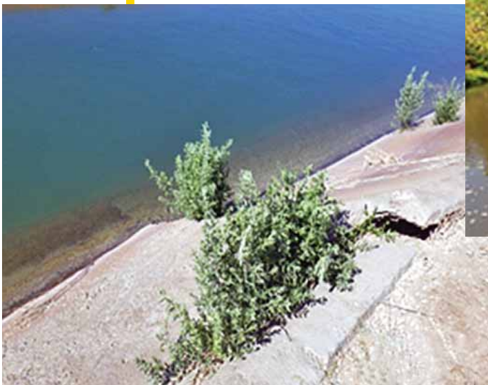
Plants growing in the joints of concrete lining and breaking the concrete panels.
