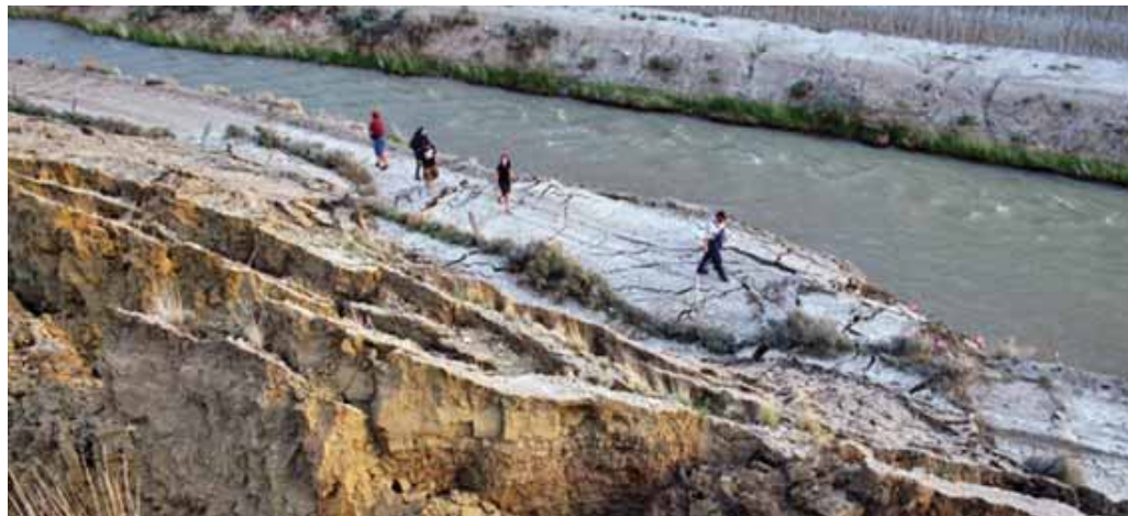
Landslides and other hazards adjacent to the canal could become active during the next rainstorm and result in overtopping in canals.
