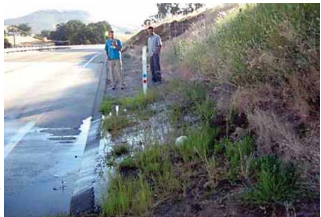
Seepage from a canal into the road below.
