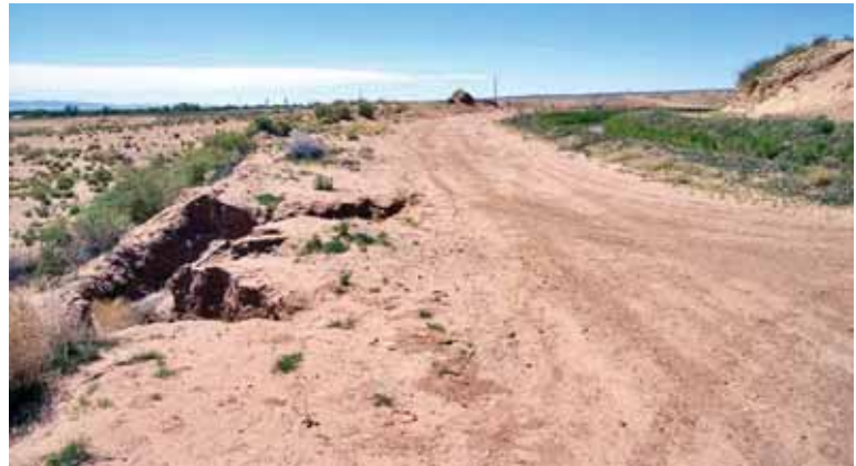
Rain channel from intense rain erosion.
