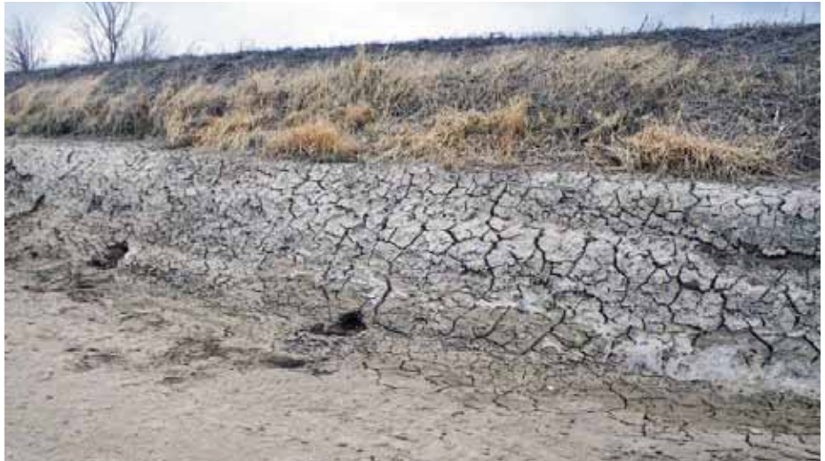
Shrinkage cracks on the inner embankment.
