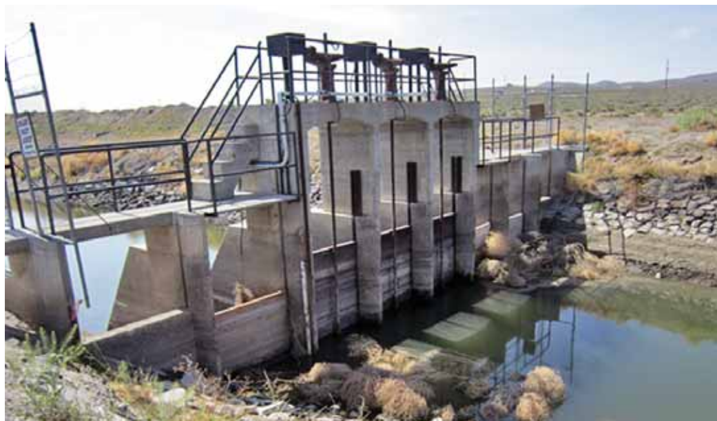
Typical check structure with gates and stoplogs.
