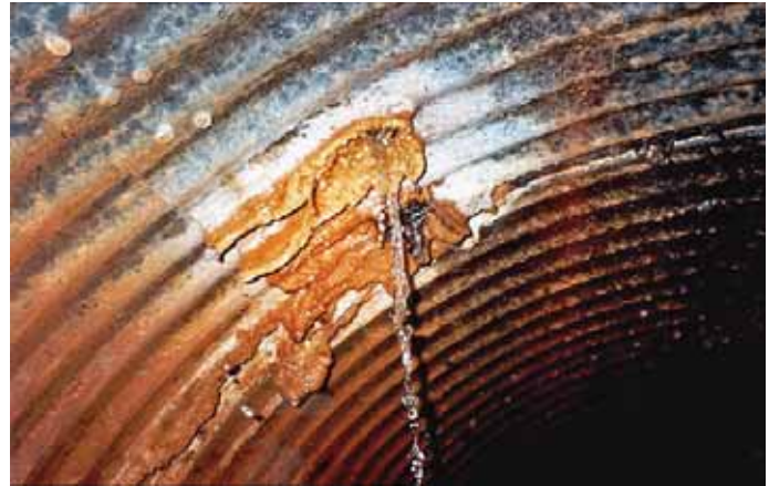
Seepage entering a corrugated metal pipe (CMP) conduit through a defect.
