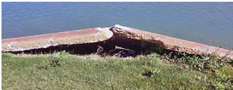
Damaged canal lining.
