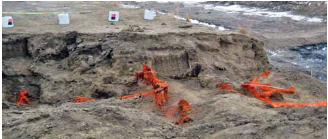
Example of rodent burrows through the embankment.
