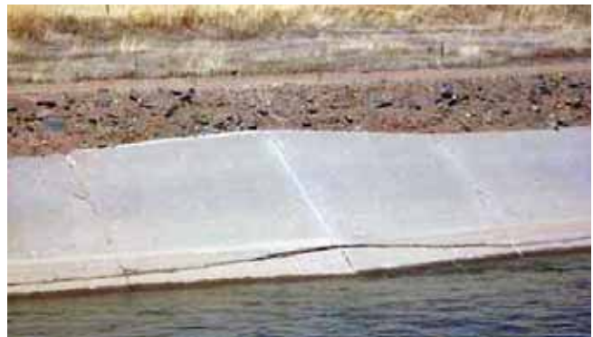
Buckle in concrete canal lining.
