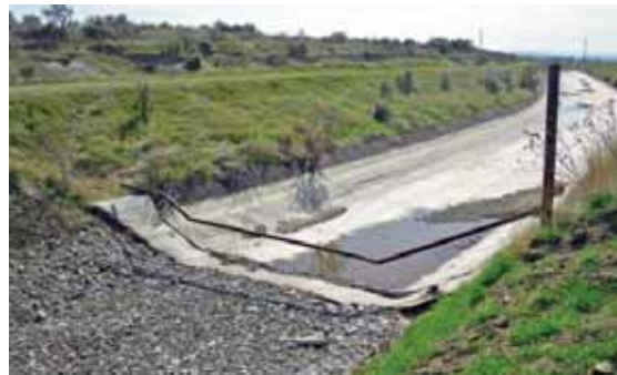
This "gate" was installed to prevent all-terrain vehicles from entering the canal.
