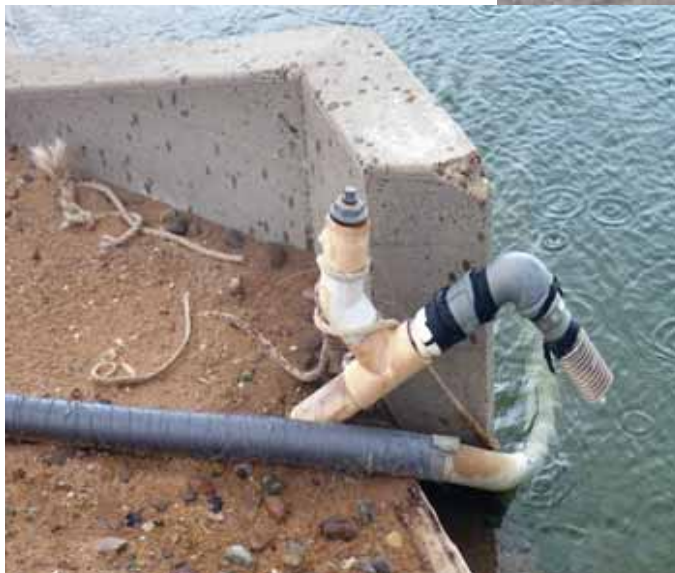
Unauthorized suction line (left).
