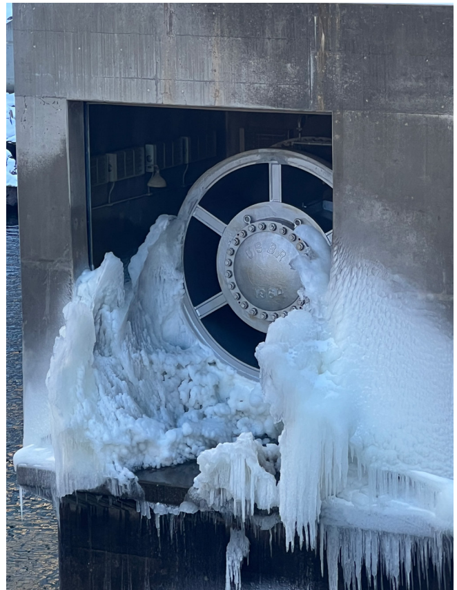
Freezing in and around hollow jet chamber of the Blue Mesa Powerplant (Colorado) bypass works during 2022 outage.
