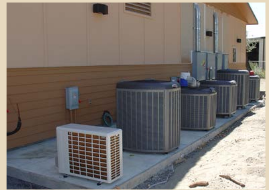
Umatilla Field Office building HVAC equipment, Hermiston, Oregon.
