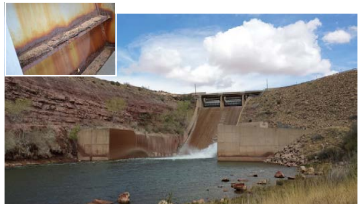
Sumner Dam, Sumner Lake, New Mexico. Inset image is close-up of rusted radial gates.
