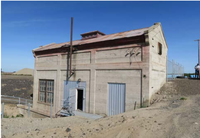
Sunnyside Canal Mile 50.35 Turbine House, Sunnyside Valley Irrigation District, Washington.
