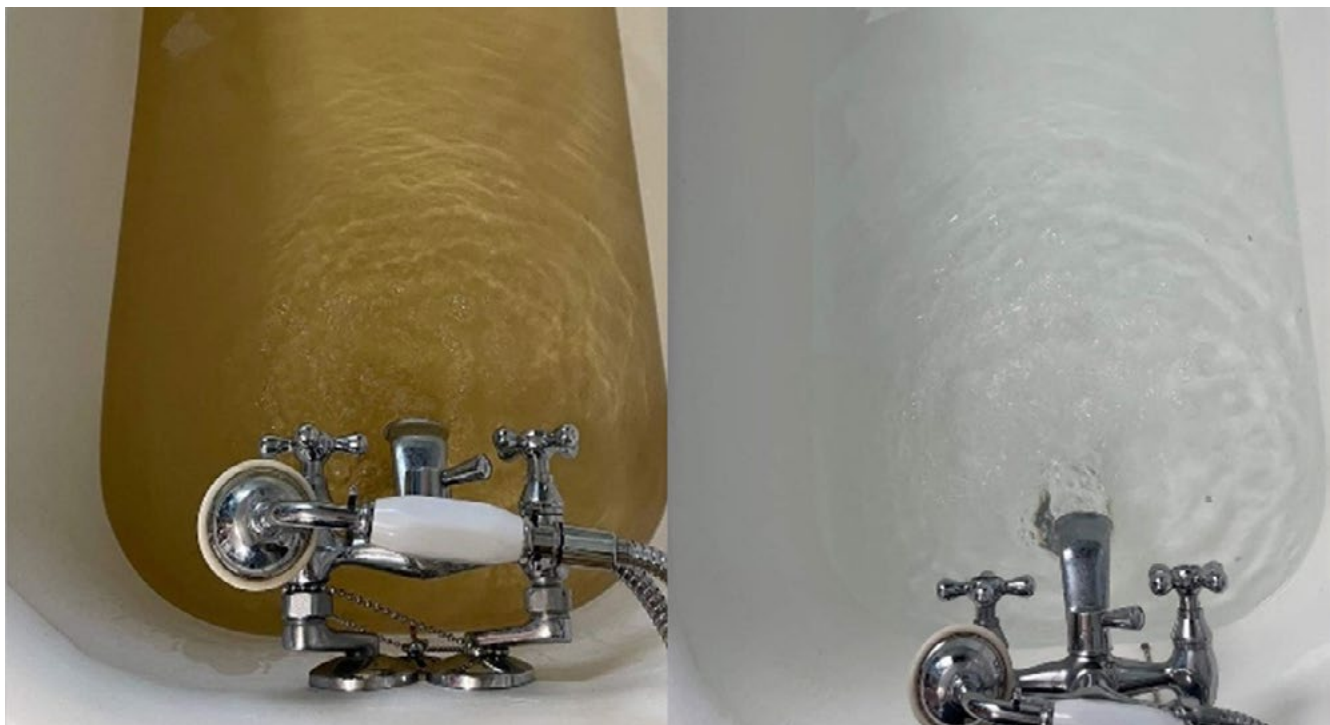
Before and after picture sent in by a mother of two, a new rural customer of Fort Peck Reservation – Dry Prairie Rural Water System, who received water in October 2022 as part of the Scobey-Flaxville Ph2 Branchline Project.
