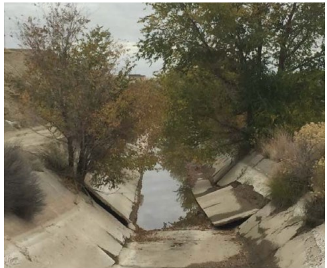
Extensive damage from trees on a concrete-lined canal.
