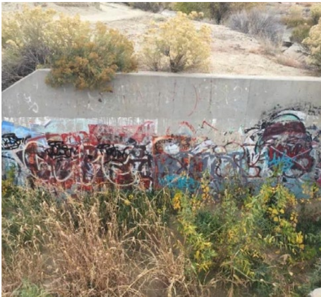
Weeds in a wasteway blocking emergency flows.
