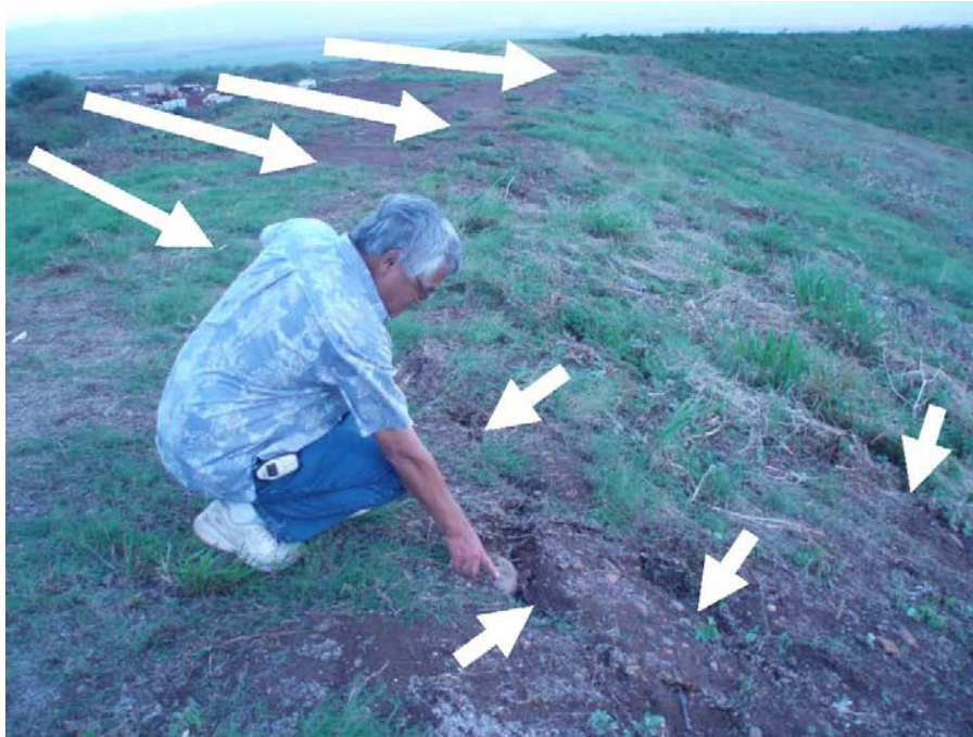
Photo 29.—Kehalani Offsite Retention Dam – Earthquake-induced cracking and sloughing (short arrows) on the upstream shoulder of the dam located about 20 feet left of the cracking shown in the previous photograph, facing the right abutment from about 20 feet to the right of the left end of the crest. Long arrows denote the 150-foot-long crack on crest shown in previous photograph.
