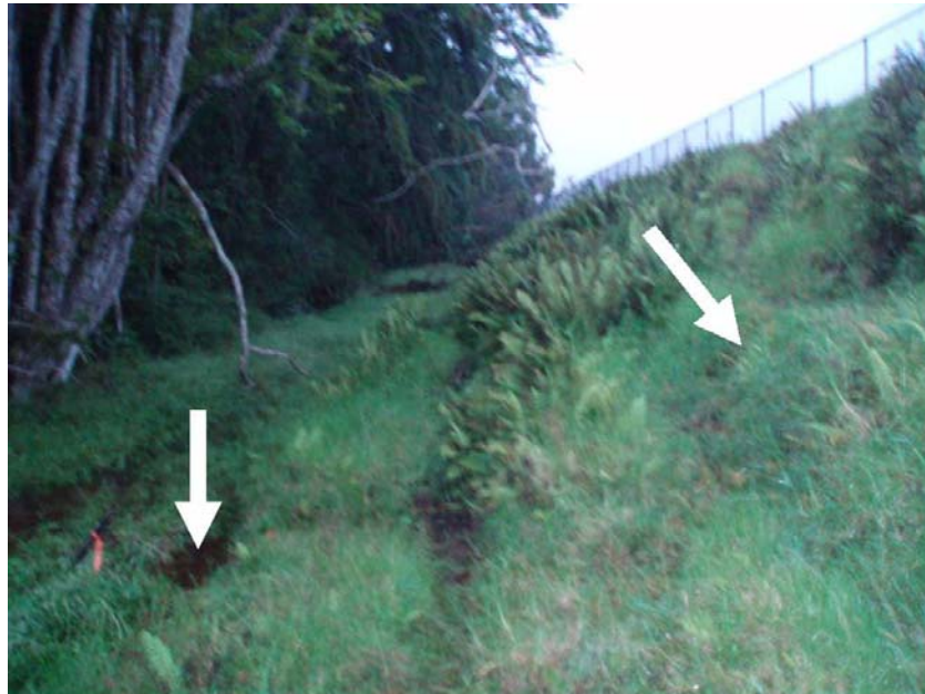
Photo 10.—Waikoloa Reservoir I Dam – Earthquake-induced sandboil area (left arrow) at the downstream toe of the dam. Right arrow denotes the downstream face of the dam. Dam is 17.5 feet high at this location. Photograph is blurry due to low light conditions and rainfall.
