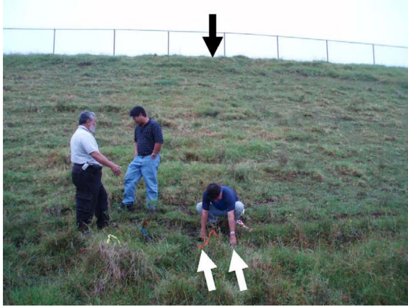
Photo 7.—Waikoloa Reservoir II Dam – Two earthquake-induced new sandboils (lower arrows) at the downstream toe of the dam shown in the previous photograph, facing upstream. Upper arrow denotes crest of Reservoir II Dam.
