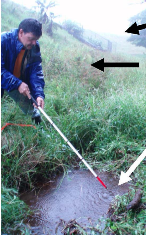
Photo 11.—Waikoloa Reservoir I Dam – Earthquake-induced sandboil area (lower arrow) at the downstream toe of the dam with three sandboils. Middle arrow denotes the downstream face of the dam, upper arrow denotes downstream face of Reservoir II Dam.
