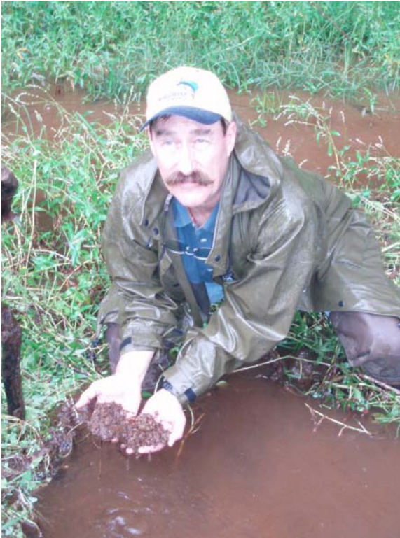
Photo 14.—Waikoloa Reservoir I Dam – Sandboil area shown in previous photographs, prior to lowering the reservoir. Inspector is collecting and examining soil materials from the earthquake-induced sandboils. The three sandboils are flowing at a total combined visually estimated rate of about 30 to 40 gallons per minute, with transported soil particles in suspension and accumulated around the sandboils.
