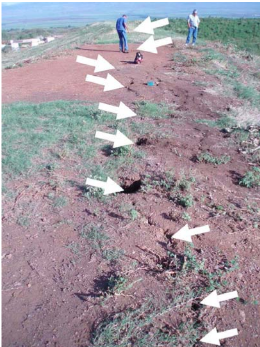
Photo 28.—Kehalani Offsite Retention Dam – Crest of the dam facing the right abutment from 40 feet right of the left end of the dam. Arrows denote a 150-foot-long, 10-inch-deep earthquake-induced longitudinal crack on the crest that starts at 40 feet to the right of the left end of the crest. Note the 12-inch-diameter, 10-inch-deep holes along the crack.
