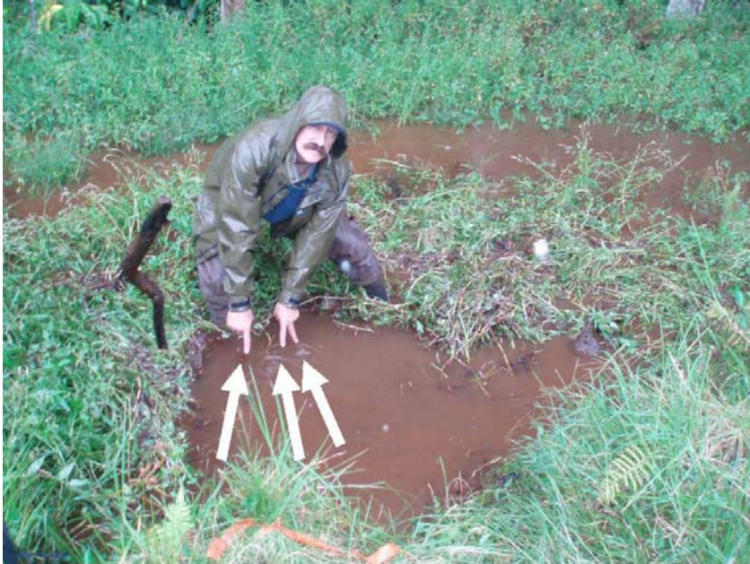
Photo 12.—Waikoloa Reservoir I Dam – Sandboil area (arrows denote three sandboils) at the downstream toe of the dam, facing downstream. Three sandboils are flowing at total visually estimated rate of about 30 to 40 gallons per minute, with soil particles suspended and accumulated around the sandboils.
