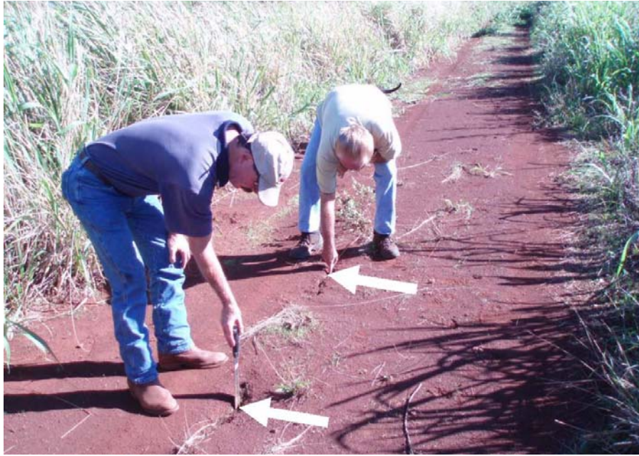
Photo 26.—Hanakoo Dam – Closeup view of the right end of the 60-foot-long crack (arrows) shown in previous photograph. Note the machete inserted into the crack at lower arrow.
