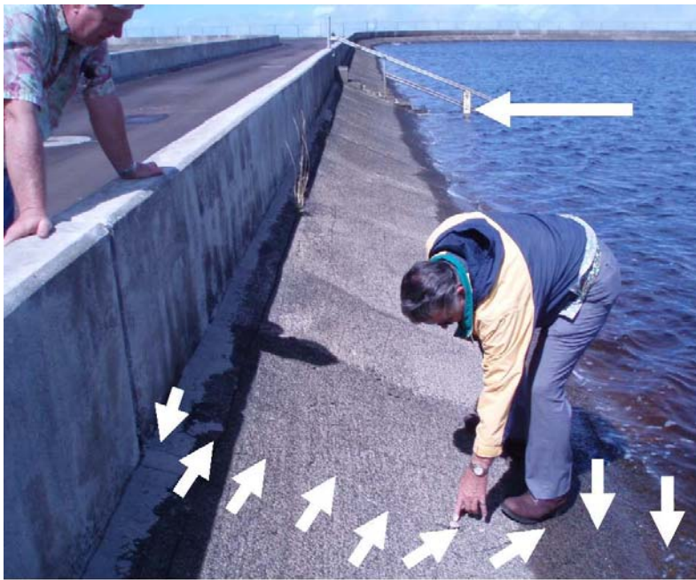
Photo 24.—Kahakapau Dam – New earthquake-induced crack (short arrows) in the concrete lining of Reservoir No. 2 facing downstream. The crack is located 55 feet upstream from the reservoir water surface elevation staff gage (long arrow).
