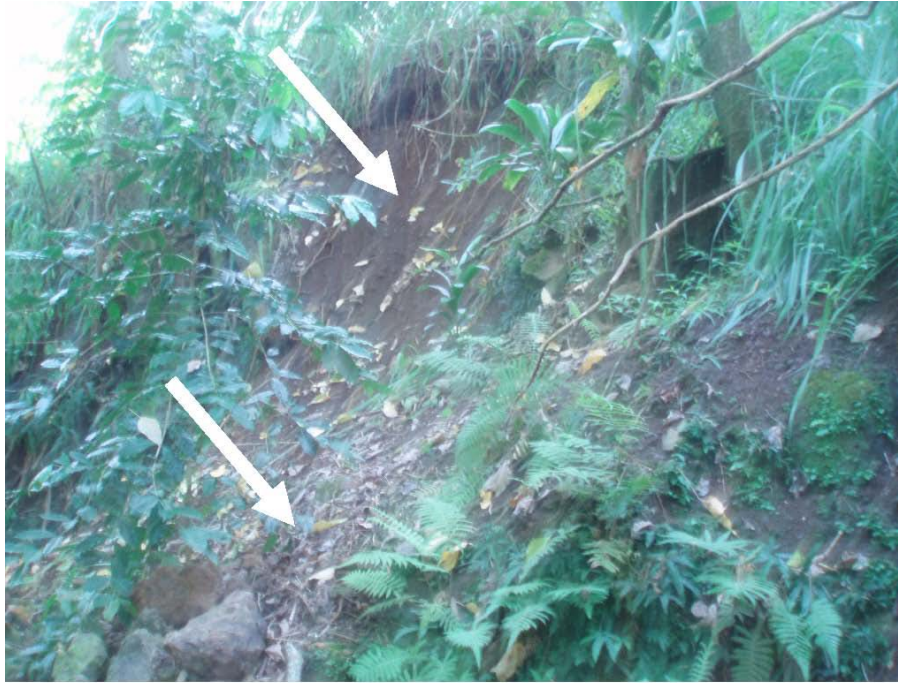
Photo 20.—Paauilo Dam – Typical earthquake-induced new rock and soil slide area (arrows) on the open cut side slopes of the spillway discharge channel. 10/18-19/2006
