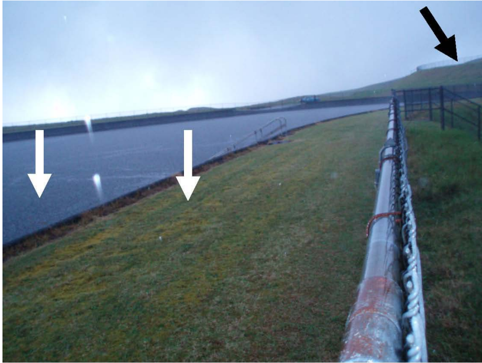
Photo 15.—Waikoloa Reservoir I Dam – Crest of Reservoir I Dam with cracking (middle arrow). Right arrow denotes Reservoir II Dam crest. Note the reservoir concrete lining parapet (left arrow). The Reservoir I sandboils are located at the downstream toe about 20 feet to right of photograph.
