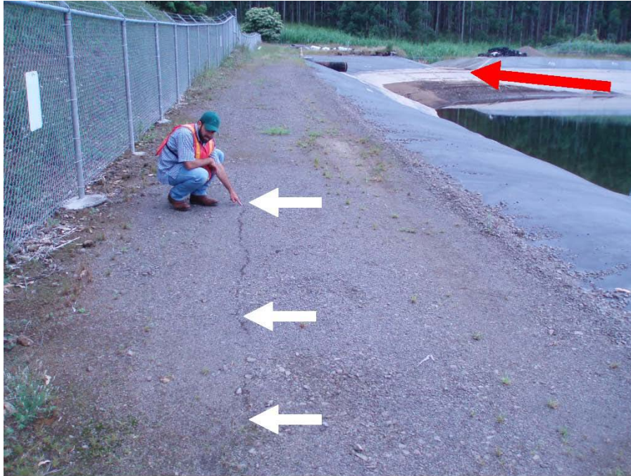
Photo 18.—Paauilo Dam – Short arrows denote the alignment of the new 25-foot-long earthquake-induced crack located 220 feet to the left (facing downstream) of the spillway. The long arrow denotes the spillway.
