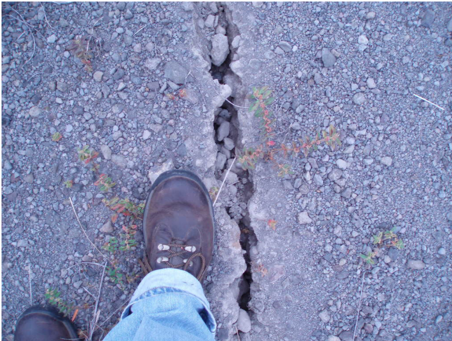
Photo 17.—Paauilo Dam – Closeup view of the new crack shown in previous photograph, with a maximum surface width of about 4 inches.
