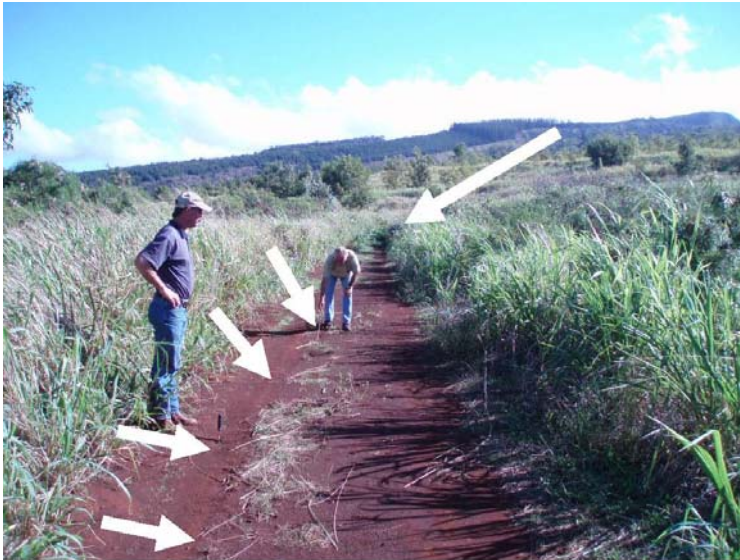
Photo 25.—Hanakoo Dam – Right end (short arrows) of a 60-foot-long, 4-foot-deep earthquake-induced crack (probed 4 feet with coffee tree stick, crack could be deeper) on the crest of the dam facing the right abutment. Coffee tree stick is slender and stiff, good for probing. Right end of crack starts 50 feet to the left of the spillway (long arrow denotes spillway pipe).
