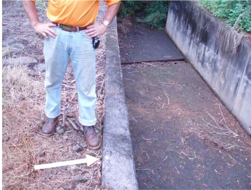
Photo 21.—Puukapu Dam – Minor earthquake-induced separation (arrow) between the backfill and right concrete wall of the Puukapu Watershed Canal facing upstream. The separation is earthquake-induced damage 15 feet long, 0.25 inch wide, and of unknown depth. This is the only location where separation is evident at the canal. The damage is about 300 feet upstream from the dam. 10/20/06
