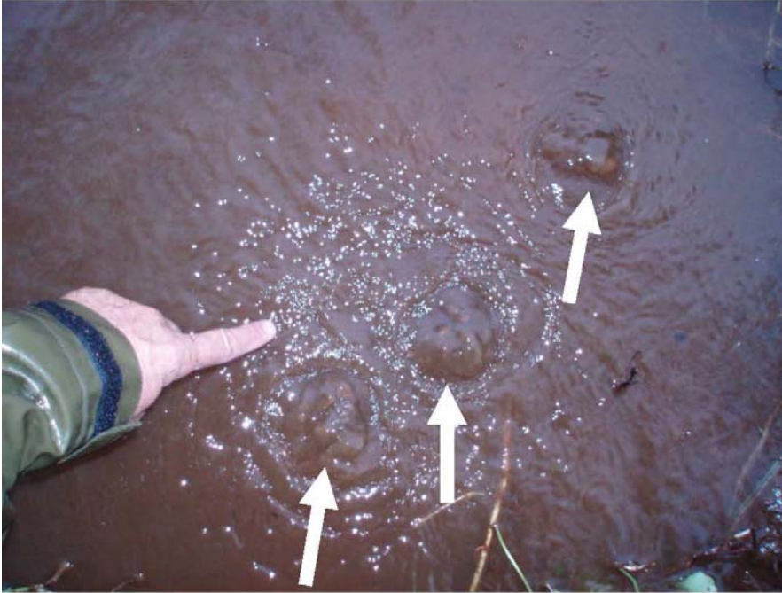
Photo 13.—Waikoloa Reservoir I Dam – Closeup view of the three sandboils (arrows) shown in the previous photograph. Note soil materials in suspension (arrows) in the rising flow from the sandboils breaking about 1 inch above the pond surface.
