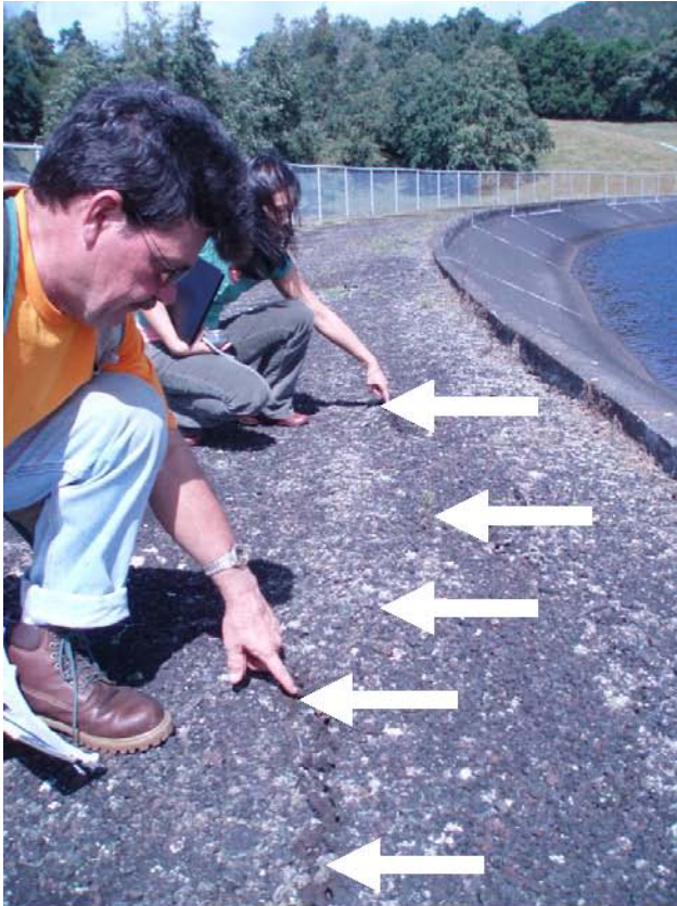
Photo 1.—Waikoloa Reservoir II Dam – Earthquake-induced new longitudinal crack in the dam crest (arrows denote alignment). Note new bulging of the crest in the area of the crack caused by earthquake shaking of the dam. Numerous other new longitudinal cracks and bulged areas are evident on the dam crest.
