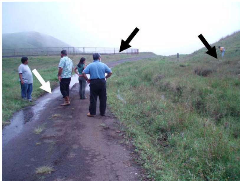
Photo 6.—Waikoloa Reservoir II Dam – Two earthquake-induced new sandboils (right arrow) at downstream toe of Reservoir II Dam. Note ponded water inundating the paved access road (left arrow) between Reservoirs I and II. About 10 percent (1 gallon per minute) of sandboil seepage was flowing into the ponded water, and 90 percent was flowing into southwest drainage area in background of photo located between right and middle arrows. Note Reservoir I Dam (middle arrow).
