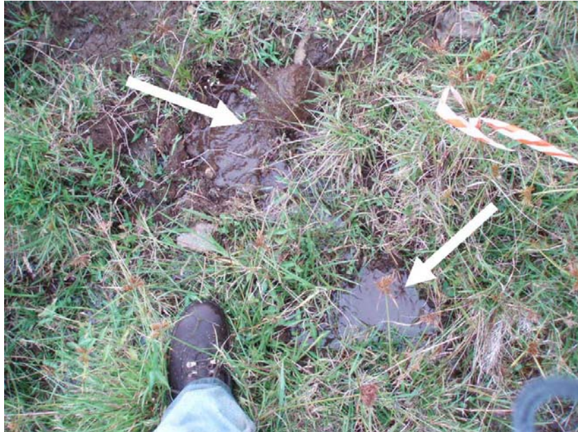
Photo 8.—Waikoloa Reservoir II Dam – Closeup view of the two earthquake-induced new sandboils (arrows) at the downstream toe of Reservoir II Dam flowing at a total visually estimated rate of about 10 gallons per minute, shown in the previous photograph.
