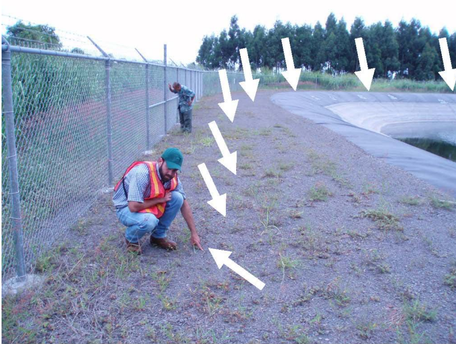
Photo 16.—Paauilo Dam – Lower arrow denotes the left end of the new 460-foot-long earthquake-induced crack (bottom arrow) located 135 feet to the right (facing downstream) of the spillway. Arrows denote the alignment of crack around the corner of the reservoir.
