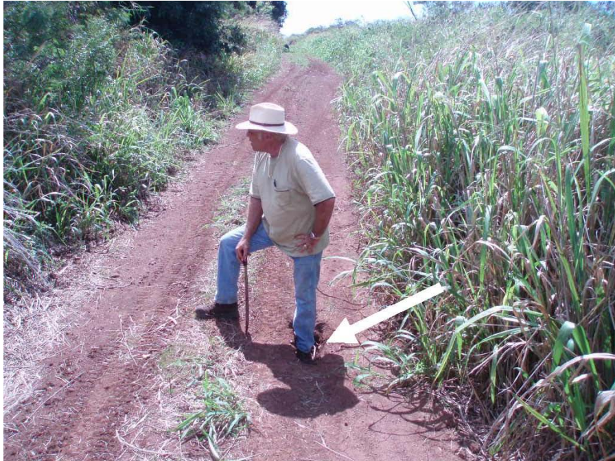
Photo 27.—Horner Dam – 2-foot-long, 1-foot-wide, 2-foot-deep sinkhole (arrow) on crest of dam of the left basin (dry reservoir) facing the left abutment. Sinkhole is 108 feet to the left of the berm dividing the left and right basins of the reservoir. 10/26/06
