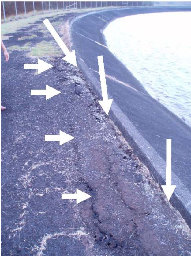
Photo 2.—Waikoloa Reservoir II Dam – Earthquake-induced new longitudinal crack in the dam crest (short arrows denote alignment). Note new bulging (area between long arrows and short arrows) of the crest paving caused by earthquake shaking of the dam and the 1-inch wide separation (long arrows) between the reservoir concrete lining parapet wall and the crest embankment material. Numerous other new longitudinal cracks, bulged areas, and areas of separation are evident on the dam crest. New transverse cracks are evident at several other locations on the dam crest.
