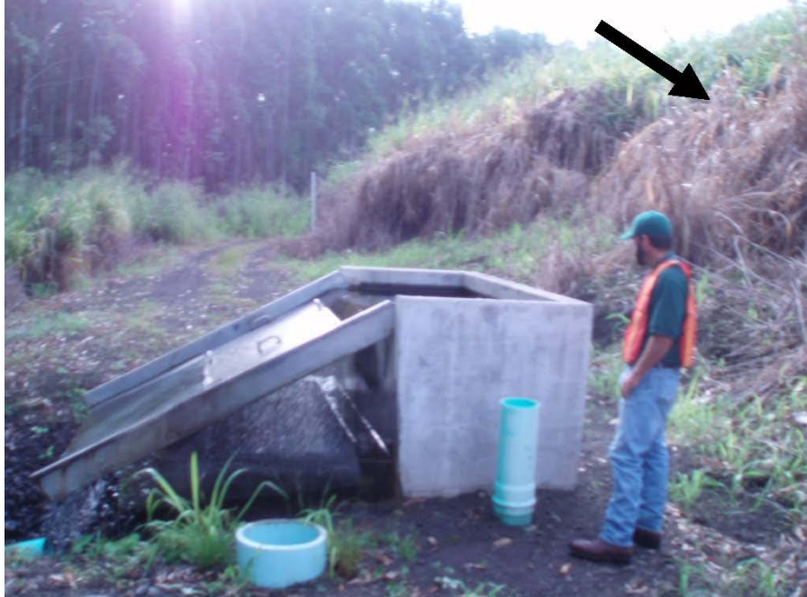
Photo 19.—Paauilo Dam – Outlet works discharge structure with no earthquake damage. Arrow denotes downstream face of the dam. Note significant amount of tall vegetation on the face.
