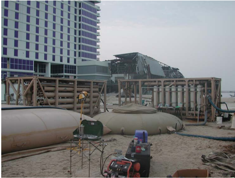
Figure 6.—Fully operational UF skid to the right, RO skid to the left, UF feed tank, and 20-kgal product storage tank and makeshift kitchen in the front.
