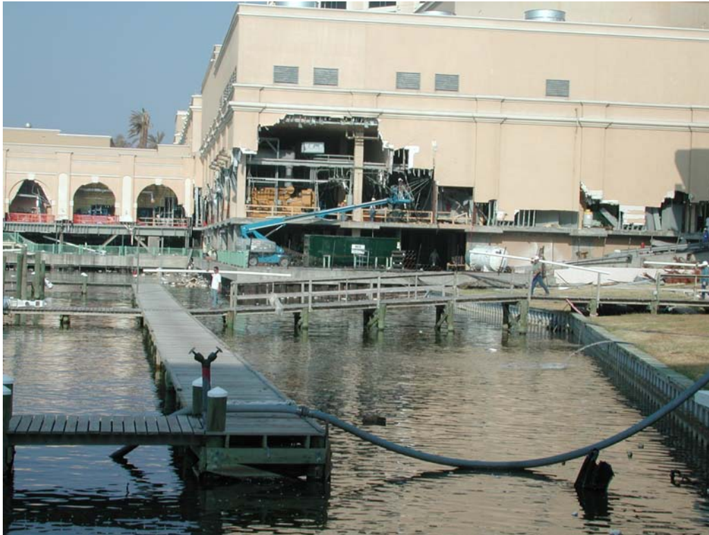
Figure 4.—Extending the intake to the end of the pier – plumbing donated by Ivey Mechanical.
