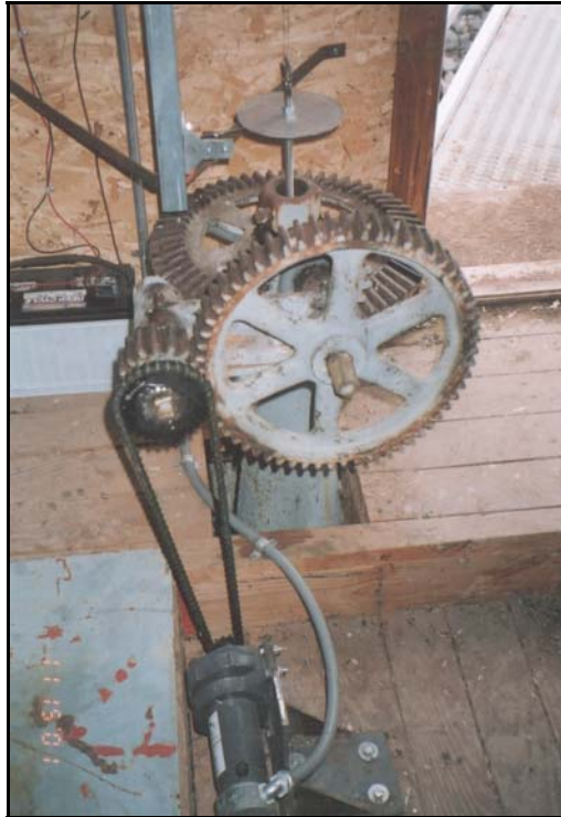
Motor- and chain-driven gear drive for operating the left regulating gate hoist.
