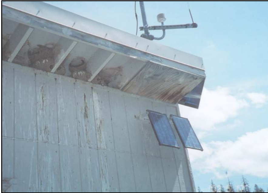
Solar panels mounted on the outside wall of the gatehouse. Bird screens are attached to the roof eave above the panels to restrict bird nesting and subsequent debris. Note the lack of organic coatings on the gatehouse siding in the vicinity of the solar panels.
