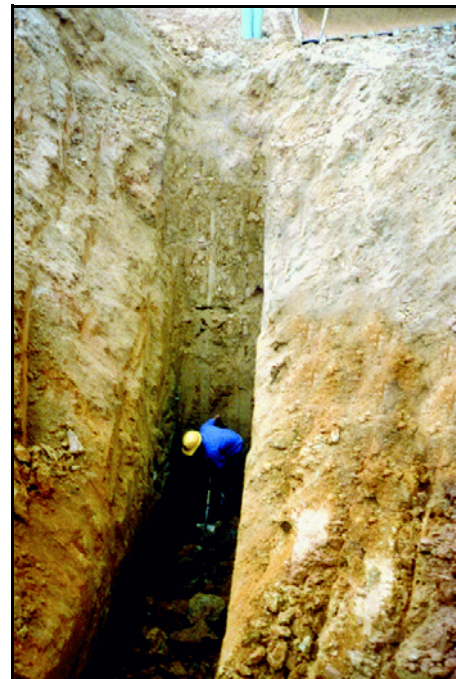
The Occupational Safety and Health Administration rates water, sewer and pipeline construction as the fourth most deadly occupation in the United States during 1999-2000. (Photo courtesy of TrenchSafety.org.)
