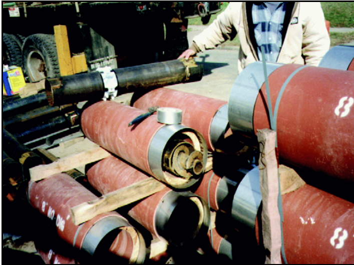
Sections of pipe await placement at one trenchless project. Increasingly, municipalities throughout the United States are specifying that contractors employ trenchless technologies for installing sewer and water lines.
