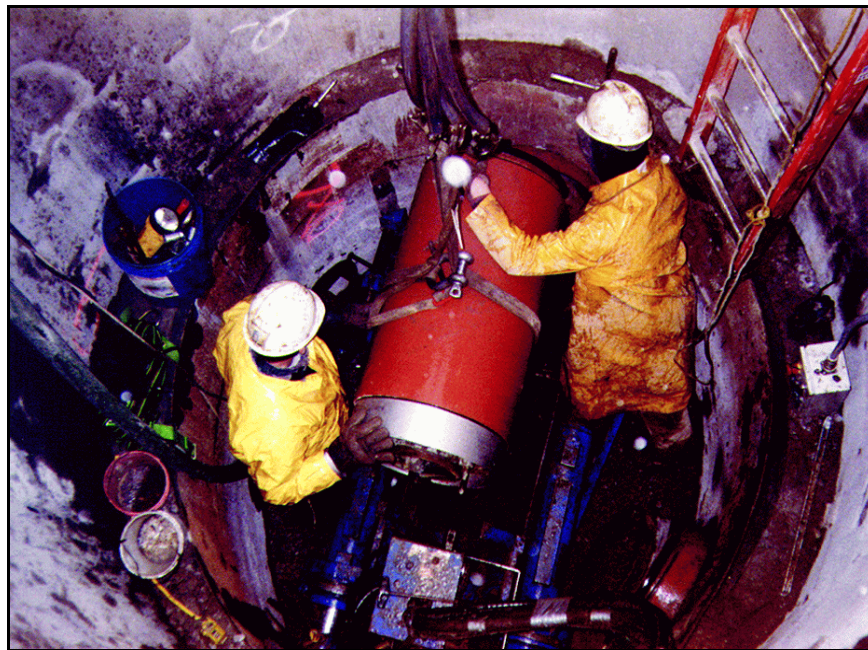
Sewer construction using pilot tube technology provides a safer alternative to open trenching.
