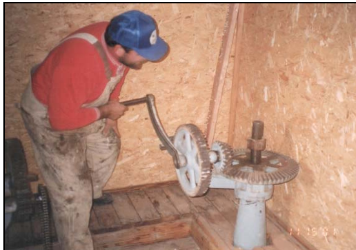
District employee enthusiastically demonstrates the proper operation of the handcrank mechanism on an emergency gate hoist.
