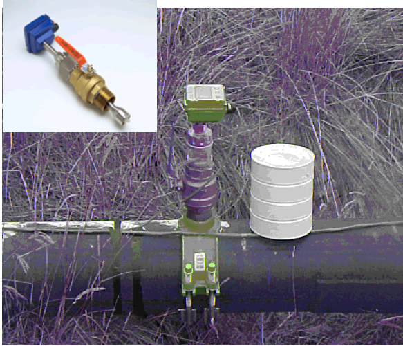
Figure 6.—SeaMetrics paddle-wheel flow meter with display installed on an 8-inch pipe. These meters may be used on pipes between 2 and 48 inches in diameter. (The white can is placed over the sensor to provide shade.)
