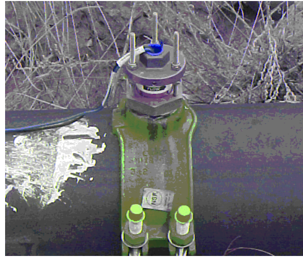
Figure 7.—Data Industrial paddle-wheel flow rate sensor installed on an 8-inch pipeline. These meters may be used on pipes between 3 and 26 inches in diameter.
