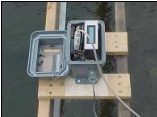
Figure 2.—View looking into the OCFR. The cable is hooked to a laptop computer for easy programming of the CPU or downloading stored data. The display shows flow in cubic feet per second and total flow in acre-feet. The ultrasonic sensor is underneath the box above the water level.
