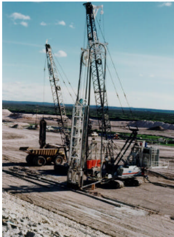
View of Casagrande hydromill, Linkbelt LS218H 100-ton crane with 30' x 10' clamshell and Cat 773 end dump truck at Primary Panel No. 277.
