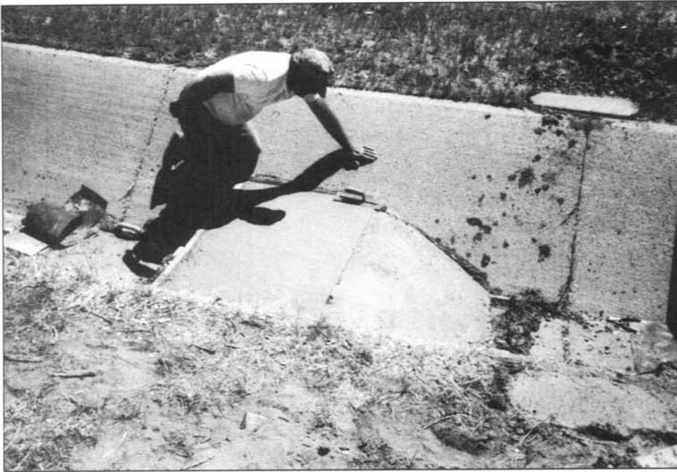
Figure 3.— Flume under construction at demonstration site NT22. The flume is 1 foot high with a 3:1 upstream transi- tion and a 2.75-foot-long throat. The 1.25:1 canal side slopes lead to a 4.5-foot-wide sill from a 2-foot bottom width.
