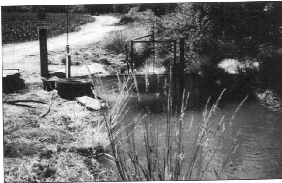
Figure 1.— Geometry upstream from demonstration site NT22 showing the check structure leading to the wasteway back to the river, the turnout, and the bridge over the farmer's canal.
