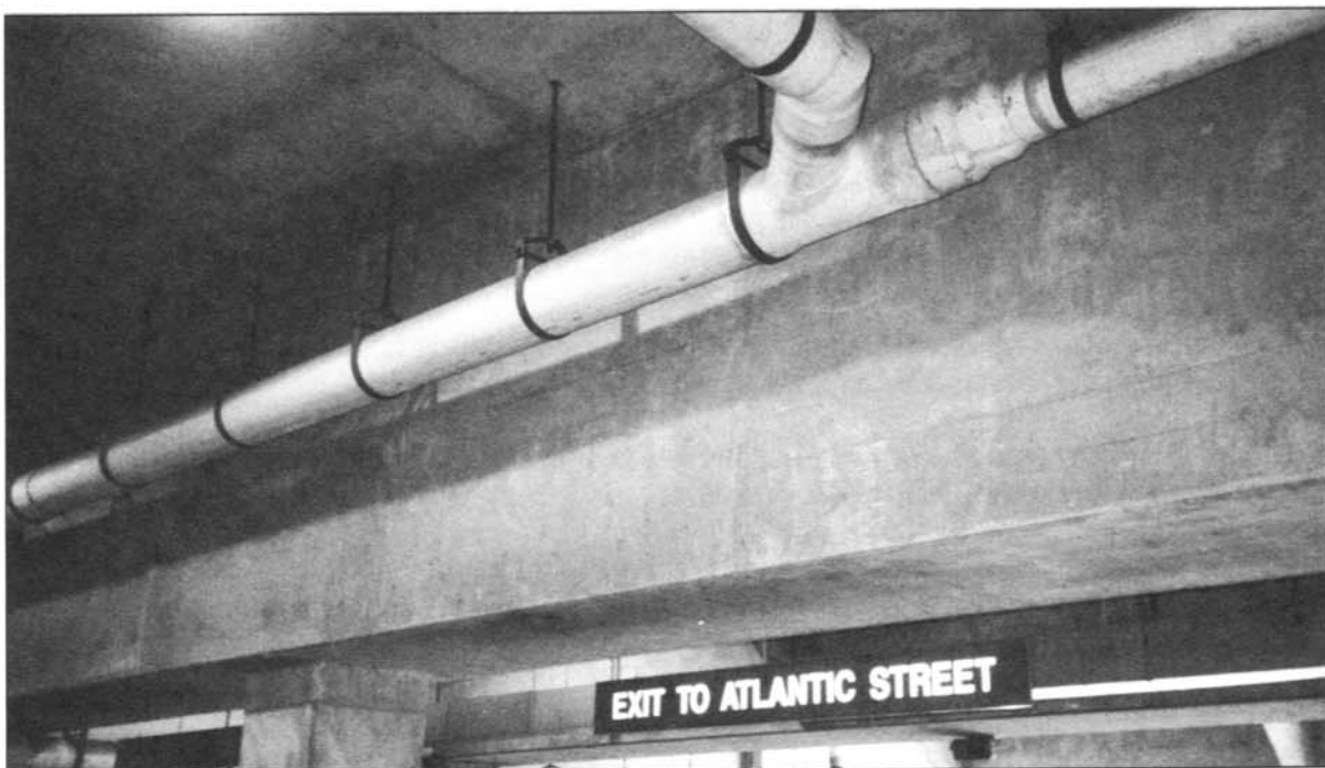
In a Norfolk, Va., parking garage, drainage is provided by this 12-inch PVC cross pipe with 10-inch piping coming from the ramp slope.
