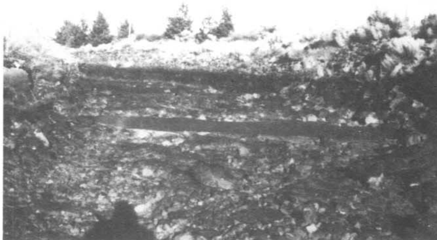
Figure 1.—Typical existing canals consist of fractured basalt bottoms with sides of loose volcanic rock.
