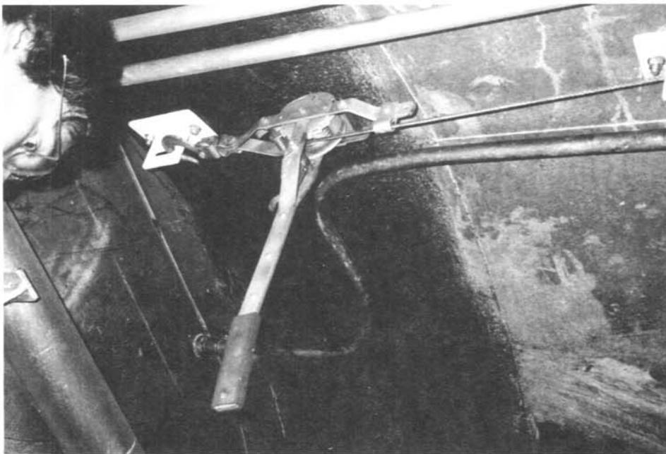
View of "come-along" hook attached to access hatch on right.
