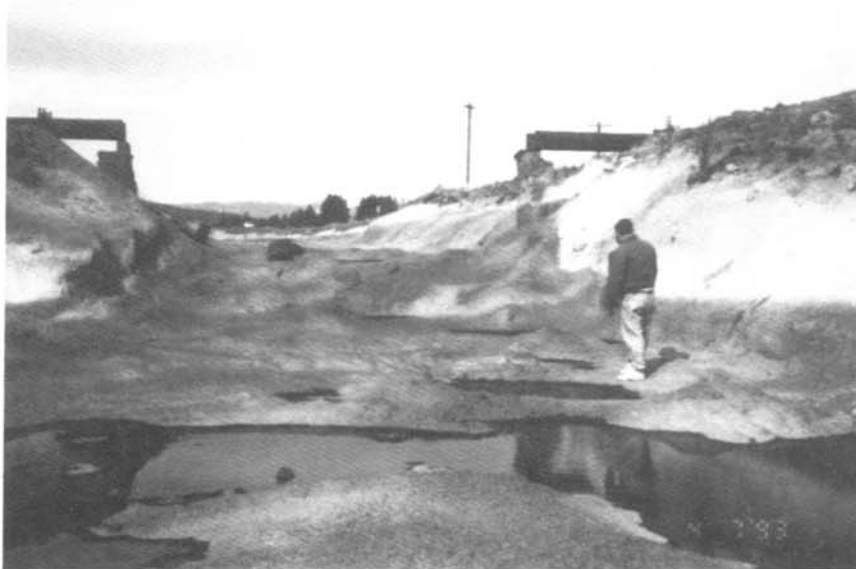
Figure 8.—North Unit Canal test sections 6 through 9. Completed canal section with 3-inch shotcrete lining.
