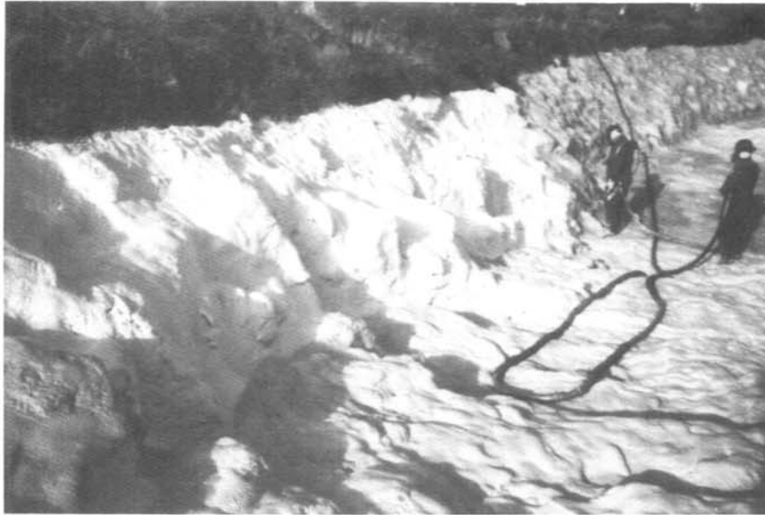
Figure 5.—North Unit Canal test sections 1 and 2. Spray application of polyurethane foam and coatings.
