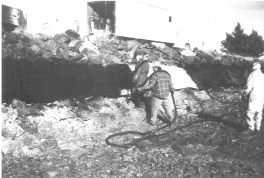
Figure 6.—North Unit Canal test sections 3 and 4. Application of protective coating to geotextile.
