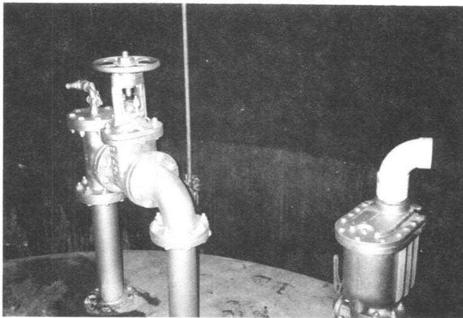
Plastic elbow installed on valve assembly.
