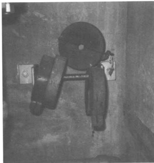
Gate valve lock covers.
