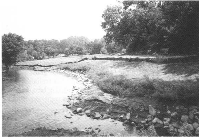
Four months after installation, willows have leafed out. Roots growing into the streambank prevent erosion and protect the bank from storm events.
