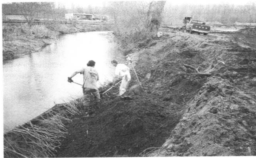
As part of an 11-acre Maryland wetland mitigation project, crew installs live willow branches in a streambank to provide bank stabilization and enhance aquatic habitat.
