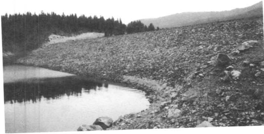
Figure 3. - Stampede Dam - Deposits of sand along upstream face of dam. 5/10/90
