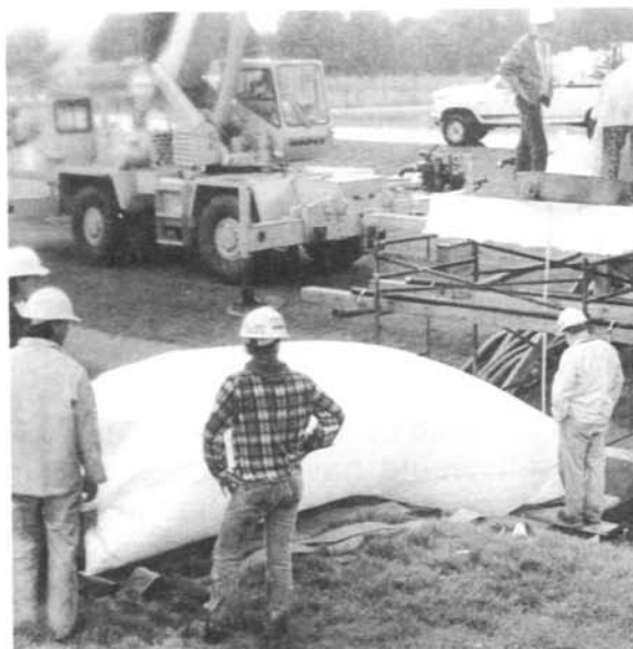
Figure 4. - Air-inflated preliner is positioned in pipe while crew works on truck platform to ready liner for placement.
