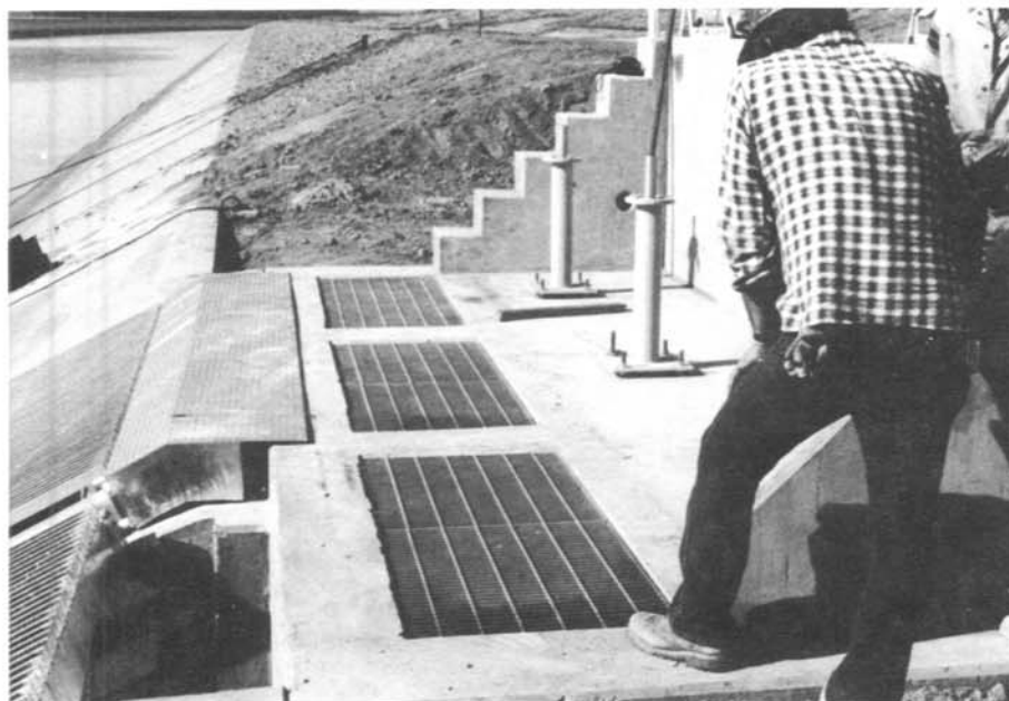
Figure 17. - View of trashracks and gratings.
