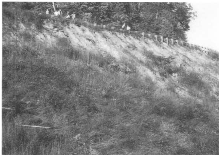
Installation of fill brushlayer during North Carolina embankment stabilization project, top; and a view of the slope before repairs began.
