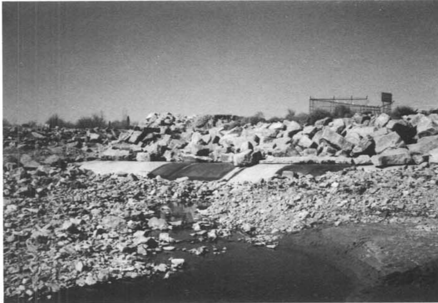
Photograph 4. – Riverside Diversion Dam. Concrete drop at downstream end of sluiceway stilling basin. 2/11/88
