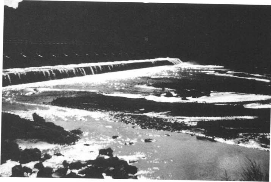
Figure 2. - Downstream view of San Acacia Diversion Dam showing depth of scour prior to rehabilitation. 11/88
