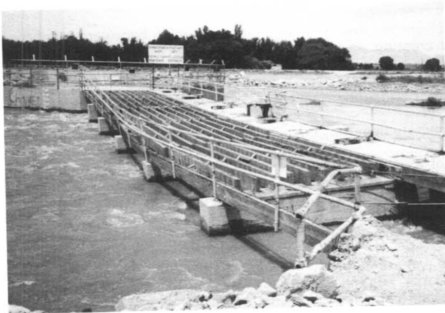
Photograph 6. - Riverside Diversion Dam. Dismantled sluiceway structure from left abutment after the failure. 7/15/87
