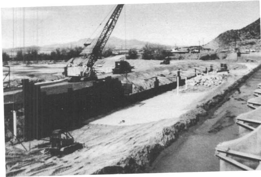
Figure 4. – Work area as viewed from the diversion dam. Some dewatering wells have been relocated to allow for geotextile placement and bedding material (center of photograph). 7/27/89
