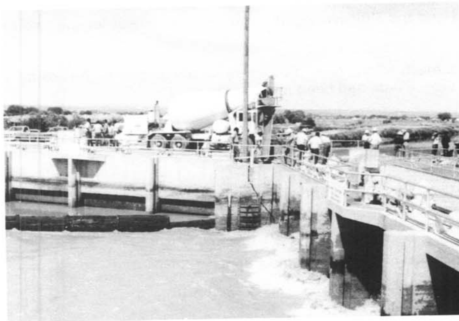
Photograph 3. - Riverside Diversion Dam. Notice crack in left upstream abutment wall of sluiceway. 6/9/87
