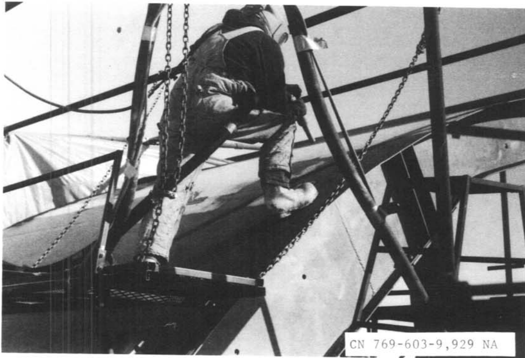
Photo 1. - McClusky Canal. Contractor is using a coal slag grit to sandblast and remove the VR-6 paint off the outside face of the south gate on Reach 3A, New Johns Lake. 3/4/89
