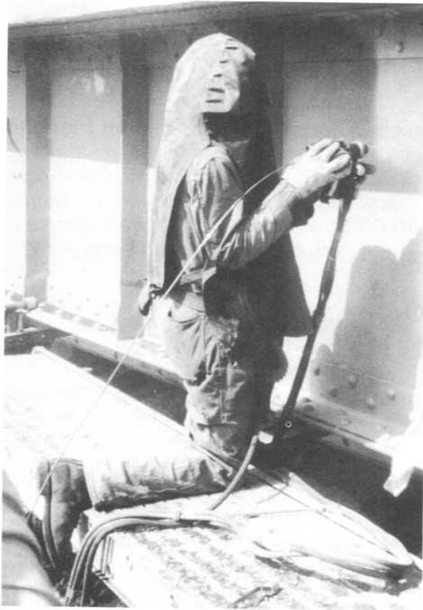
Zinc being sprayed on to the steel understructure of a bridge in Ohio; 20 years maintenance-free service is expected as a result.
