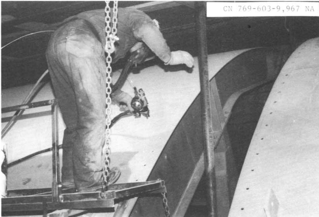
Photo 3. - McClusky Canal. Contractor applying zinc to surface to north gate. Note position of metalizing gun. 3/8/89
