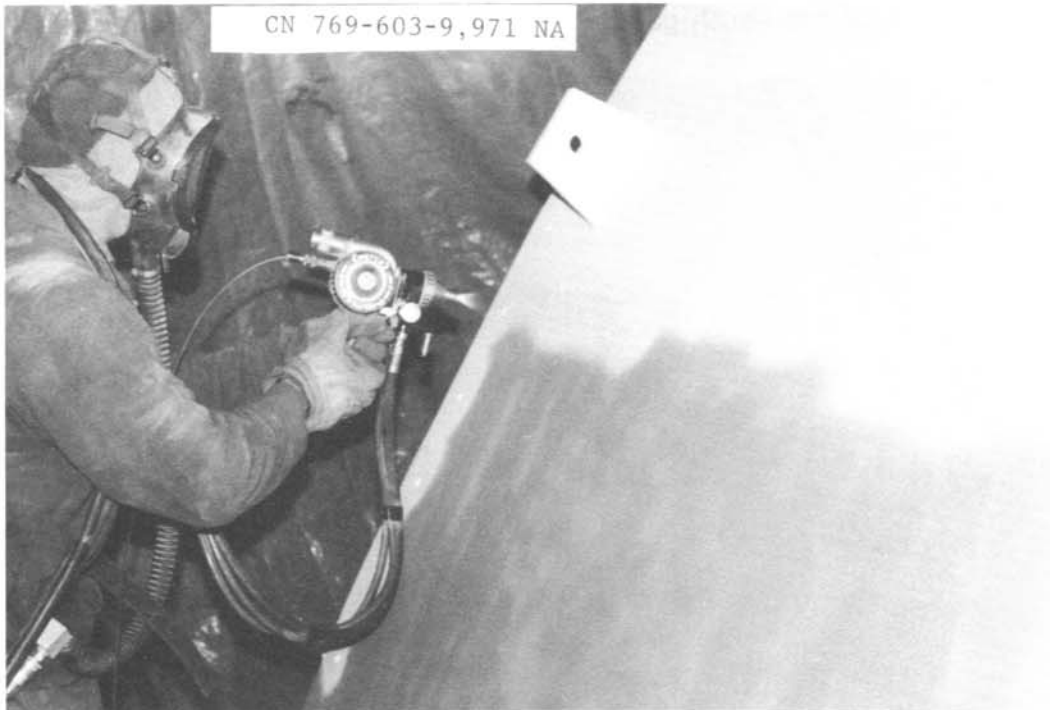
Photo 4. - McClusky Canal. Contractor applying the initial zinc coating to the 2-foot-wide section that was sandblasted just prior to metalizing. A Metco wire gas spray applicator was used to apply the zinc coating. The zinc wire is being pulled through the rear of the applicator, and the hoses attached to the bottom of the applicator supply the acetylene and oxygen.
