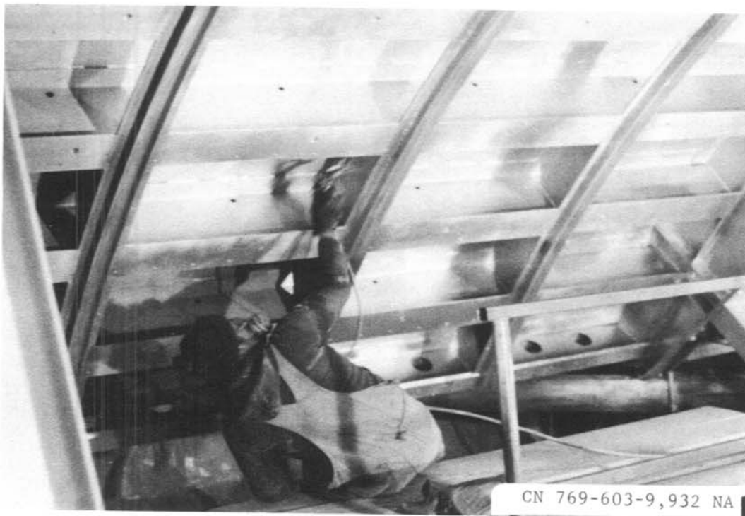
Photo 2. - McClusky Canal. Contractor is using an airless paint sprayer to apply the aluminum vinyl seal coat to the inside of the south radial gate at New Johns Lake. 3/8/89
