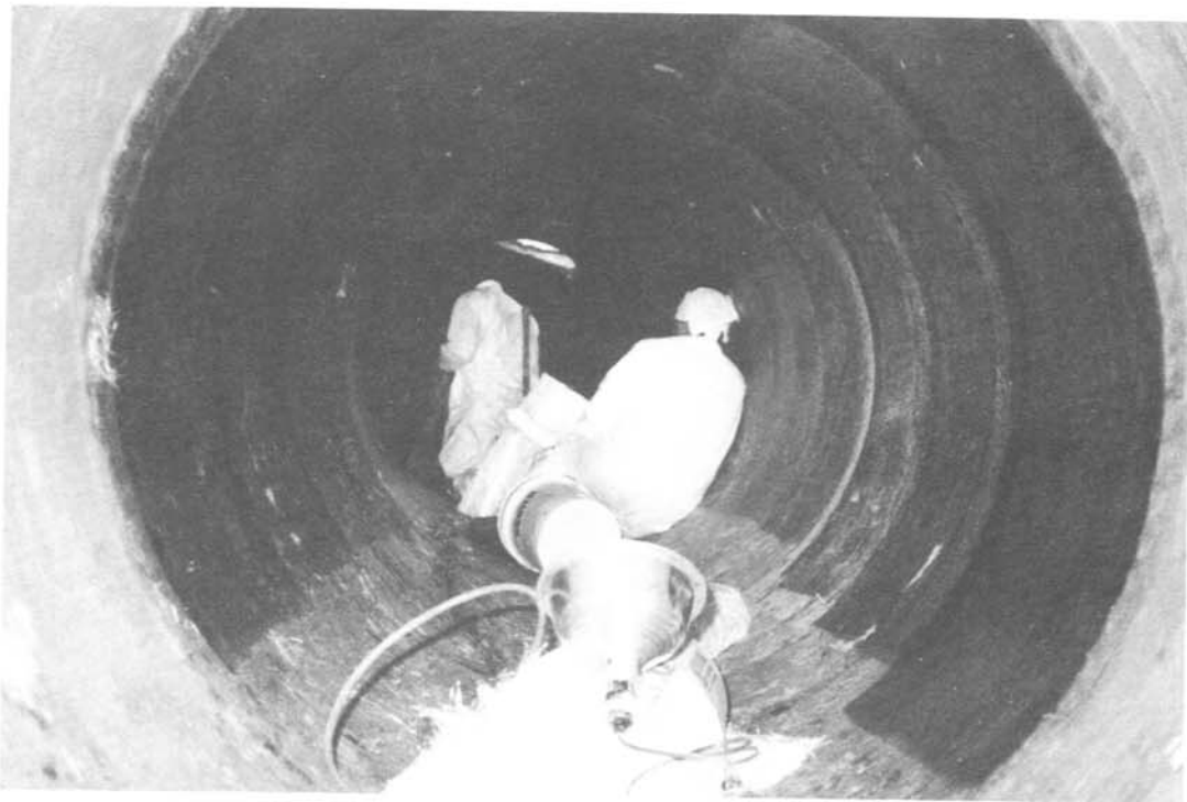
Figure 5. – Two layers of chopped mat are applied (above) and allowed to cure. After this, two top coats containing abrasion-resistant additives and wax sealers will be applied to complete the coating system.
