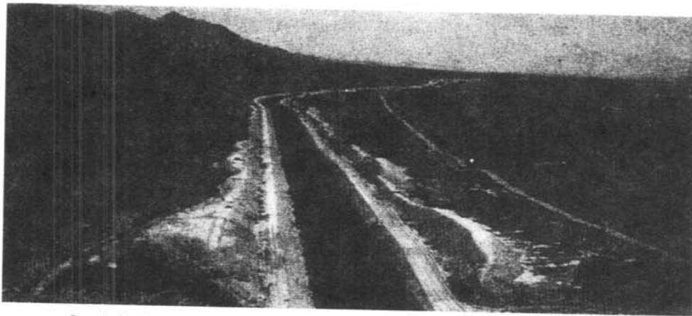
Coachella Canal in southeastern California is being relined to reduce water seepage.
