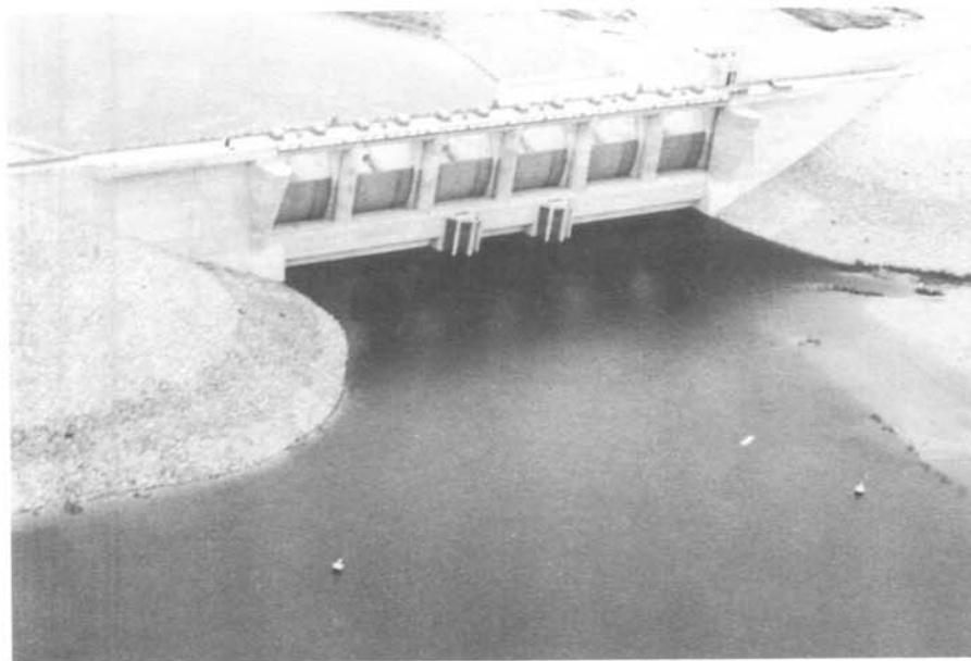
Figure 4. - Brantley Dam - Aerial view of the Reservoir and concrete structure. Note two safety buoys to which a safety float line will be connected between these buoys. 9/20/88
