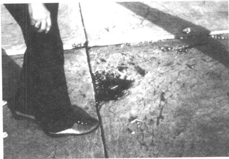
Photo No. 2. - Webster Dam - example of "D" cracking present on many slabs. 10/72
