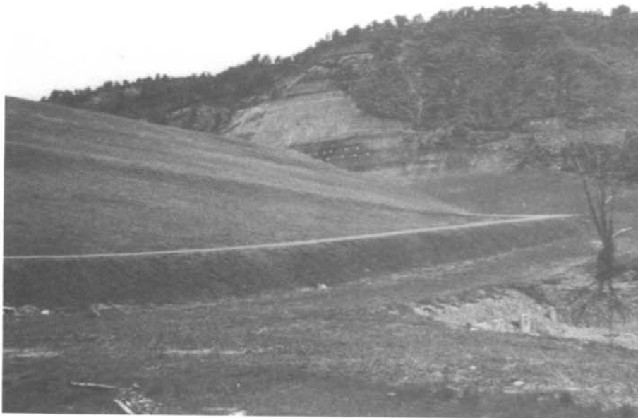
Photo 4. - The vegetation clearance zone and natural grasses on the embankment satisfy the criteria.
