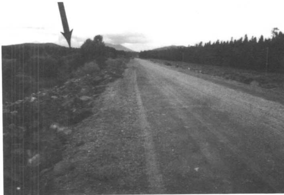
Photo 2. - Conifers and deciduous trees are established in a large area immediately upstream of the dam (arrow) and need to be removed to permit surveillance of any problems such as reservoir seepage which is known to exist.
