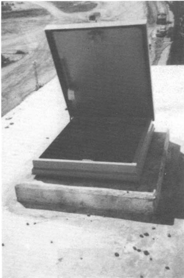
Photo 5. - Grab bars are needed to allow operating personnel to climb safely through the roof hatch.
