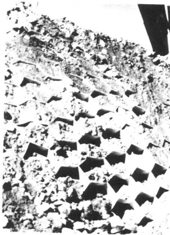
The honeycombs of the Armater were filled with a mixture of rock fine, consisting of baseball- to football-size rocks, and soil to keep the banks stable.
