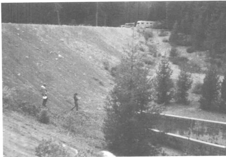
Photo 6. - Apron downstream of the toe of the embankment. The conifers on the apron are masking the stilling basin and any evidence of problems that may exist in these areas.
