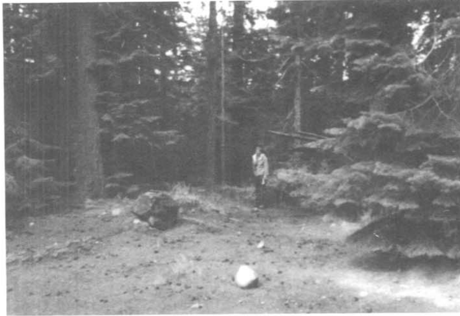
Photo 1. - The dense conifer stand has been allowed to grow in the lower end of an unlined spillway and will adversely affect and impede flood flows.
