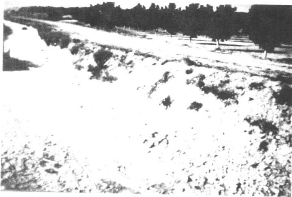
The Elephant Butte irrigation system consists almost entirely of earthen canals, laterals, and ditches.
