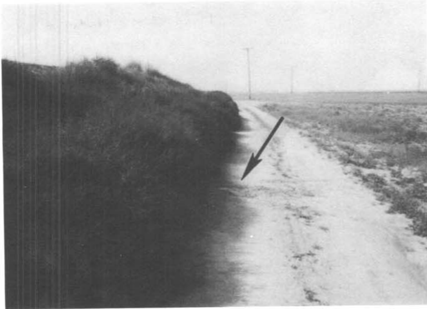
Photo 9. - The chaparral-type growth on the outside slope of the canal fill is concealing exit points of subsurface seepage channels. Material eroded from the fill has been deposited at the toe of this slope (arrow).
