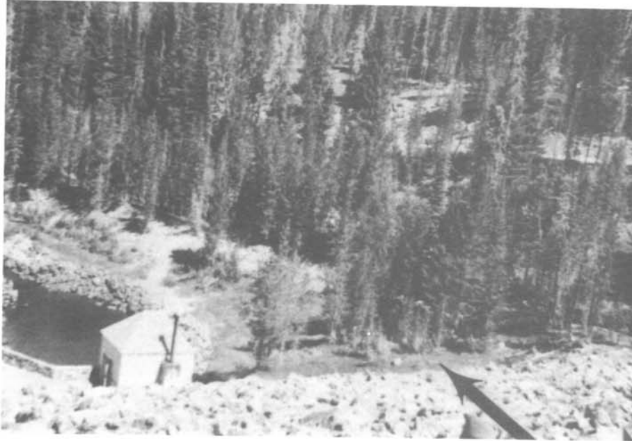
Photo 3. - Conifers have established themselves in the seepage area to the right of the valve house (arrow). They should be removed because they are partially concealing the seepage area and any evidence of adverse changes that may occur.
