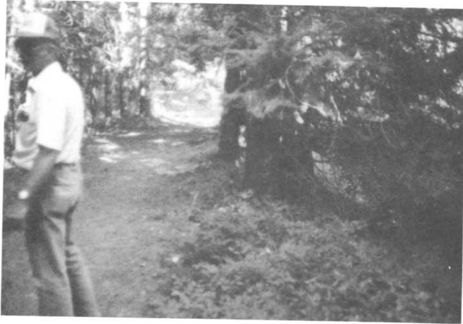
Photo 11. - Mature conifers have established themselves on both the upstream and downstream faces of this low saddle dam. Surveillance of rodent habitats and structural problems is difficult to perform.
