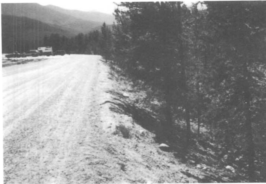
Photo 10. - Conifers have established themselves on the downstream face of this saddle dike and can conceal evidence of any problems in this area.
