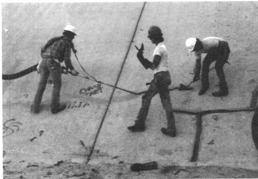
Figure 10. – Elastomeric cap-seal is tooled to correct shape with aid of a "shoe."
