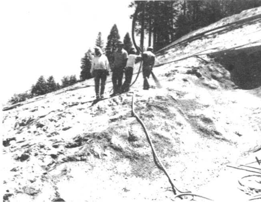
Figure 8. - Pneumatically applied concrete being placed on foundation material as protection against weathering.
