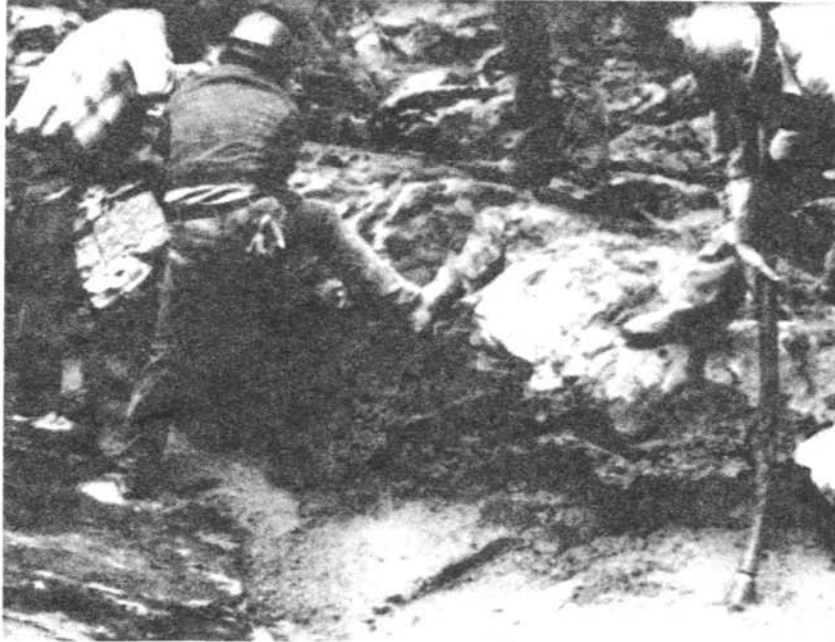
Figure 10. - Large holes in the river bottom were filled with dental concrete. Concrete was dumped from transit mixers and consolidated with a 3-inch vibrator.
