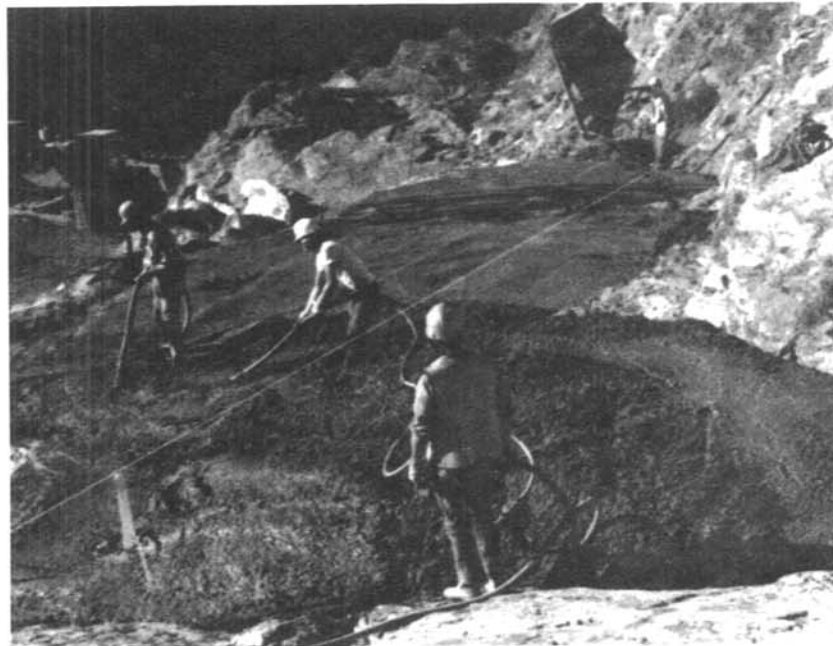
Figure 9. - Placing low slump dental concrete on a large bench along the right abutment. A crane and bucket were used for transporting and placing the concrete.
