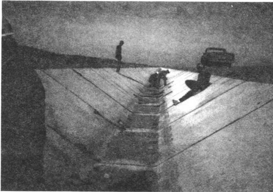
Figure 14. – Sealant is removed from the joint and replaced because of poor bond.
