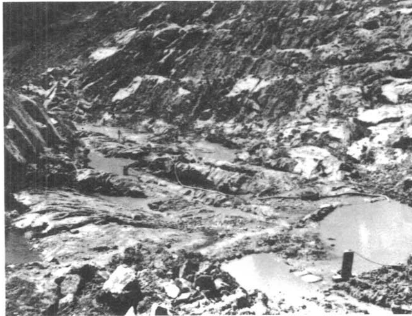
Figure 4. - A-joints on the left abutment that were nearly normal to the dam axis.
