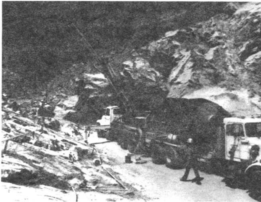
Figure 11. - Transit-mix truck delivering high slump concrete to the Thomsen 875 concrete pump. The truck boom and concrete delivery line are fully articulated and capable of rotating 360°.
