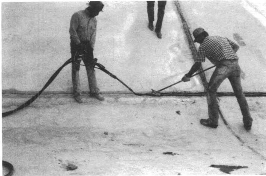
Figure 9. – Rapid-set, two-component sealant is used to seal both longitudinal and transverse contraction joints.
