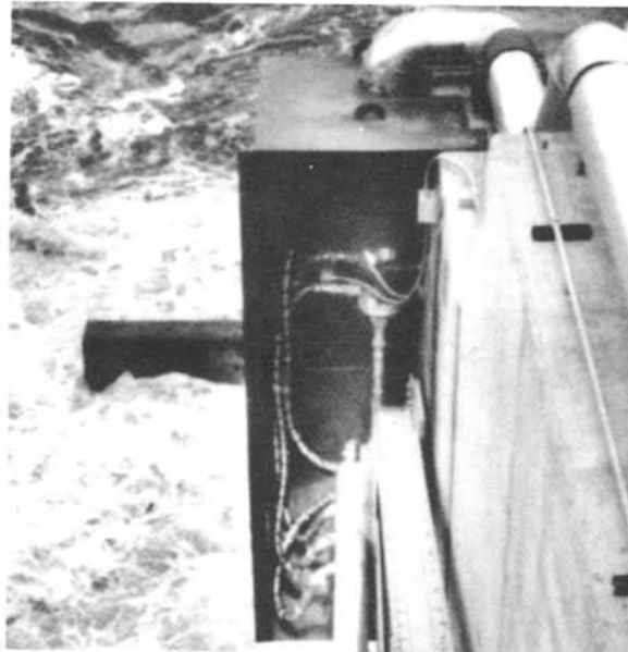
A detail view of the connection of the compressed air header pipe on the pier wall and the header on the gate arm. Flexible hosing connects the two headers and, in this application, the hosing is wrapped with heat tape. Photo courtesy of Mead and Hunt, Inc., Madison WI.
