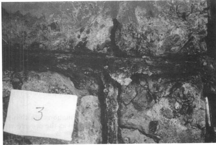
Figure 10. Underside of Sample No. 3. Steel is severely corroded and concrete is severely cracked and spalled.
