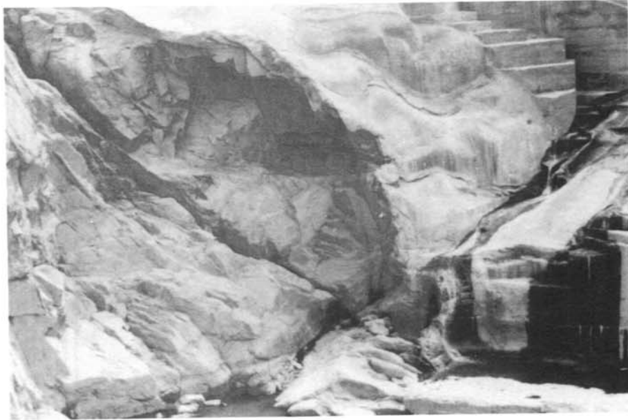
Bartlett Dam – General view of damage downstream of spillway chute. Note open joints and overhanging rock and concrete. Photo taken April 25, 1978.
