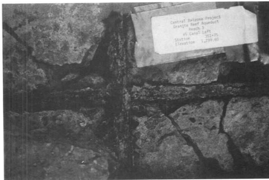
Figure 11. Underside of Sample No. 5. Again steel is severely corroded and concrete is severely cracked and spalled.
