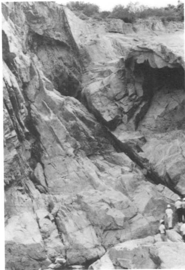
Bartlett Dam – Damage downstream of spillway chute, showing open joints and overhanging rock and concrete. Photo taken April 25, 1978.
