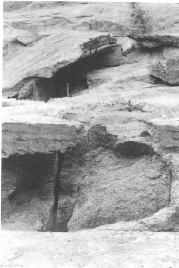
Bartlett Dam - Damage concrete and gunite and open joints in rock foundation. Photo taken April 25, 1978.
