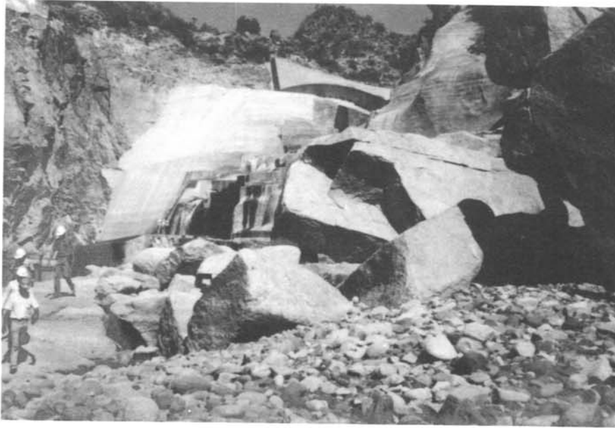
Bartlett Dam - Downstream end of spillway chute and channel armoring. Photo taken October 10, 1984.
