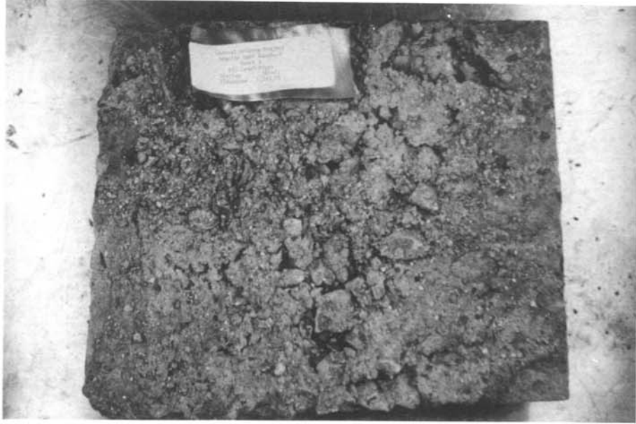
Figure 5. Bottom surface (soil side) of Sample No. 10. Concrete is not completely consolidated.
