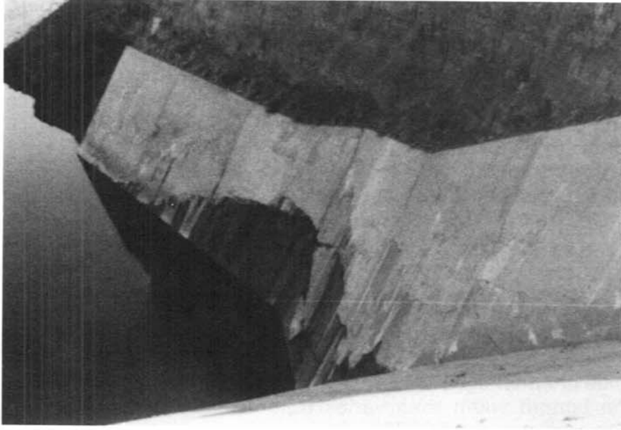
Big Sandy Dam—Cracks in stilling basin right wall. 10/8/80
