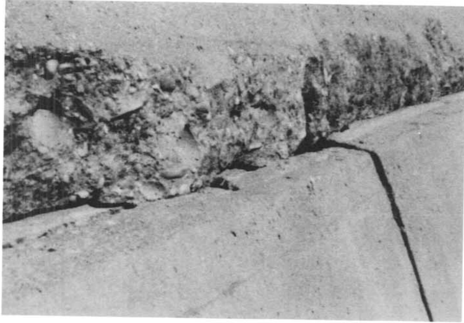
Big Sandy Dam—Spalled concrete and differential movement of spillway wall. 10/8/80
