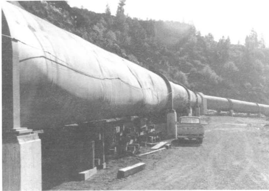
Photograph 8 - Collapse of pipeline as a result of air vent freezing or being plugged with ice during dewatering. This particular section has been replaced. (Special Note: The control cable (shown on pipeline) should be installed at the downslope side of the siphon (as shown) to prevent damage from falling rocks.)
