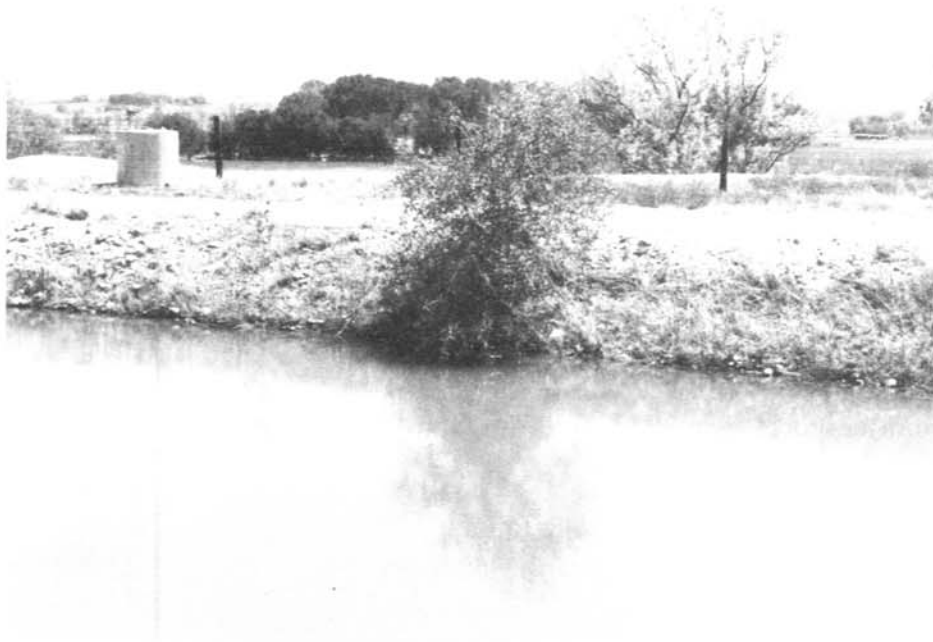
Photograph 1—Willows growing on membrane-lined ditch bank.
