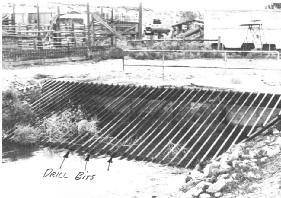
Photograph 6—A well designed and installed trashrack.
