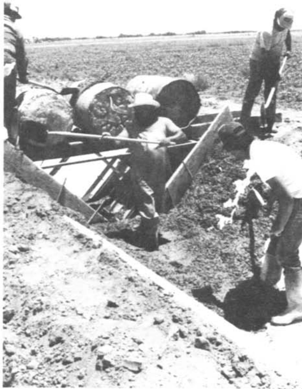
Installing a measuring flume for measuring the amount of water in a ditch.
