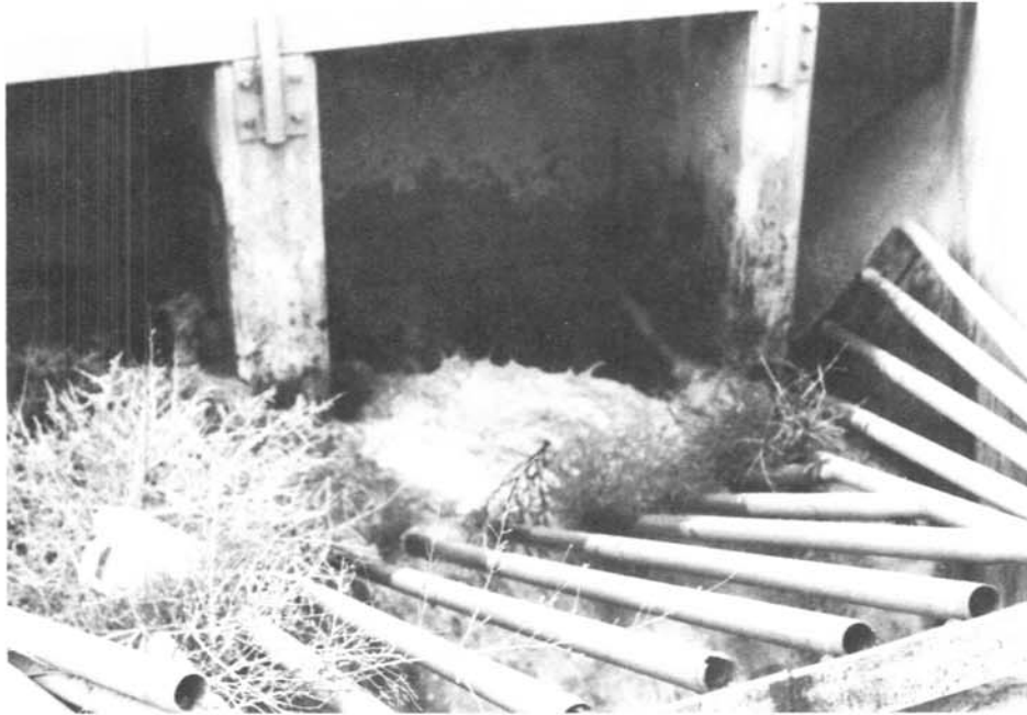
Photograph 8—A trashrack which has undesirable features (poor conformity, nonparallel members, steep, etc.).
