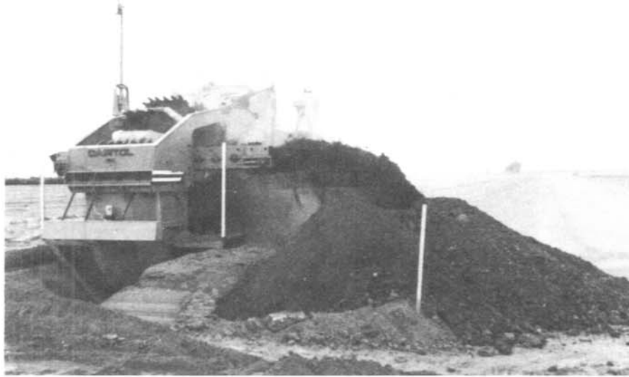
A ditch digger makes easy work of putting in a new ditch in line with a farmer's conservation plans.
