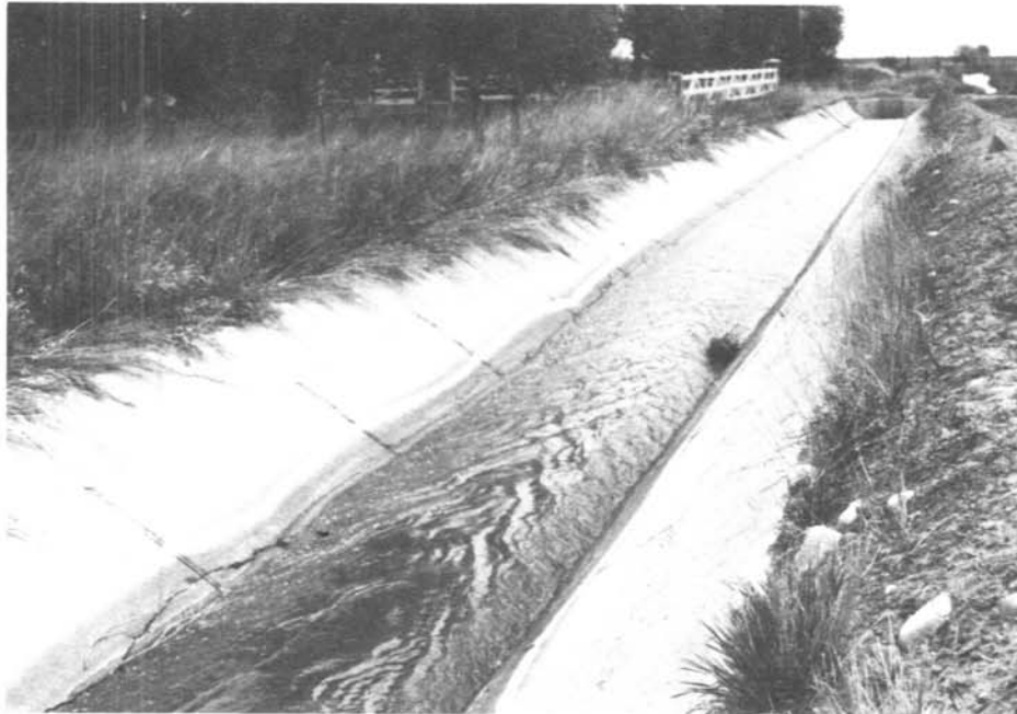
Photograph 3—Damage to concrete lining.
