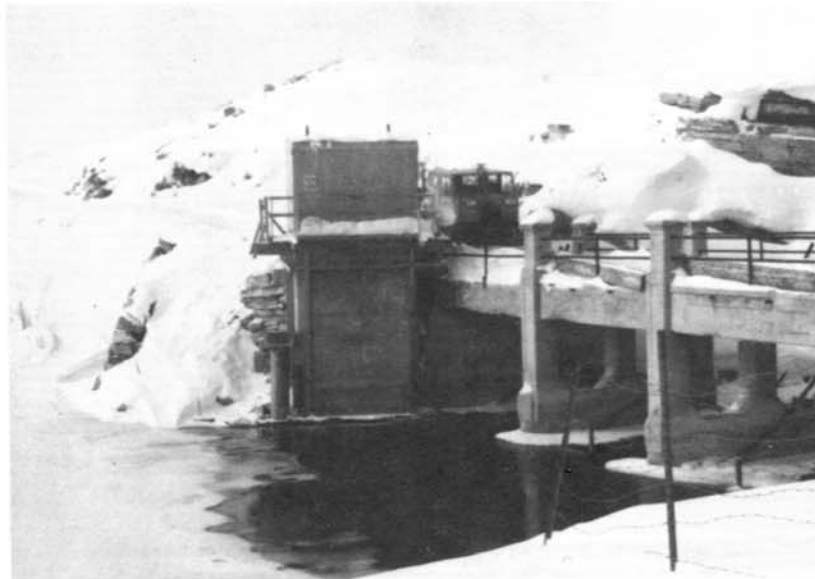
Wooden enclosure over hoisting platform. Note gate stems protruding through roof, both gates were open and water flowing through sluice tunnel.
