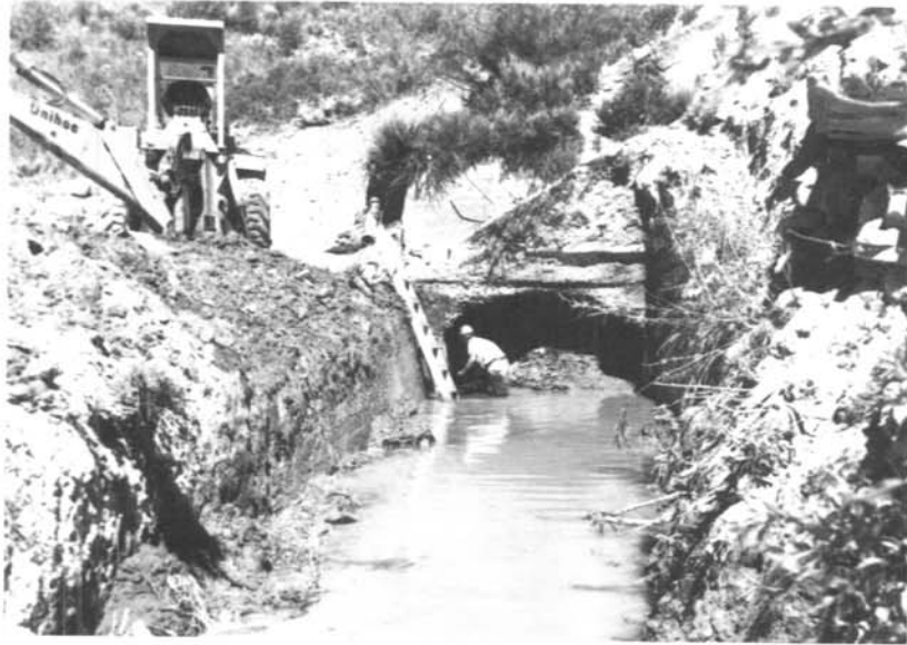
Removing earth cover at the Strawberry Dam sluice tunnel outlet portal for inspection of the sluice gates.
