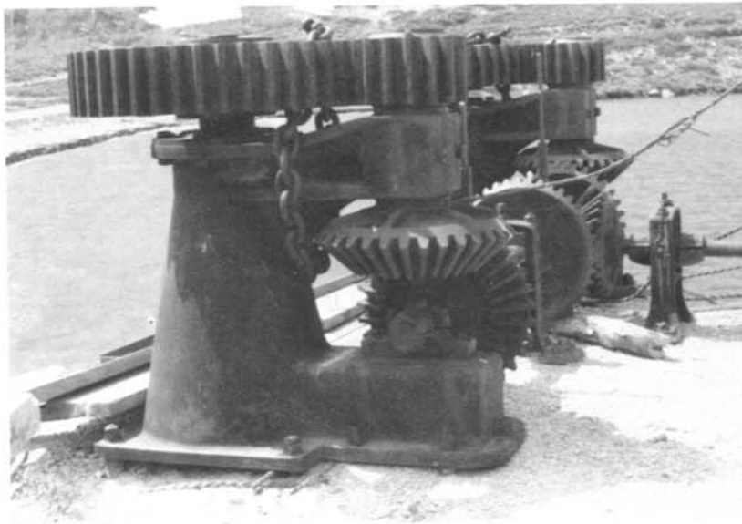
Original Strawberry Dam sluice gates hoisting mechanism. Note square twisted rebar protruding from weathered concrete.
