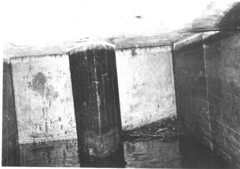
North gate (right), south gate (left), and divider as seen from downstream after water had been drained from tunnel.
