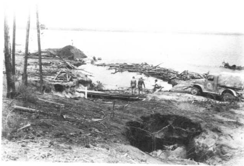
THE BIG LEAK AT BASE OF DAVIS MOUNTAIN 5-27-48—Bureau of Reclamation photo by R.A. Baker.
