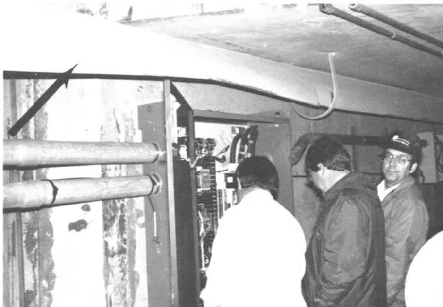
Emergency generator transfer switch located in the access tunnel was flooded. Note collapsed ventilation duct from external pressure.
