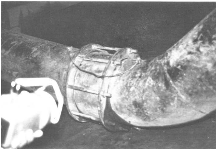
Example of dresser-style coupling unsupported for thrust load.
