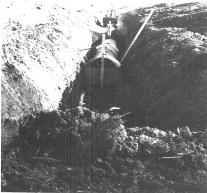
A view of main pipeline construction west of Yakima along the Tieton branch of the Burlington-Northern Railroad.
