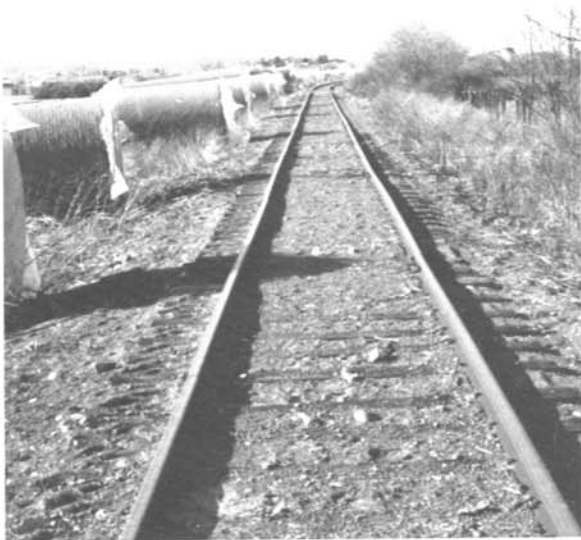
Two views of main pipeline construction west of Yakima along the Tieton branch of the Burlington-Northern Railroad in late February. Improvements on the 70-plus-year old Yakima-Tieton Irrigation District system should be completed by the spring of 1986.
