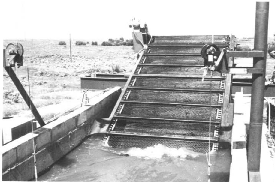
Figure 1.—Power-driven trash screen for canals and laterals.
