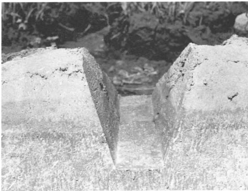
Figure 9.—The notches are formed 6 to 8 in (152 to 203 mm) deep into the freeboard and will spill freely.
