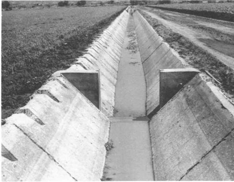
Figure 8.—Saw-toothed, laser-guided concrete ditches do not need siphon tubes for efficient water delivery.
