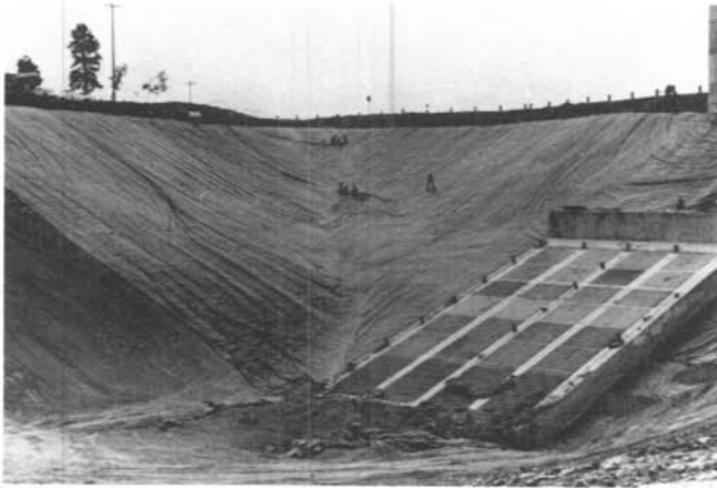
Figure 6.—Installation of CPER flexible membrane lining around inlet-outlet structure in Mt. Elbert Forebay Reservoir. After the lining was installed, earth cover materials were placed over it for protection from the elements and physical damage.
