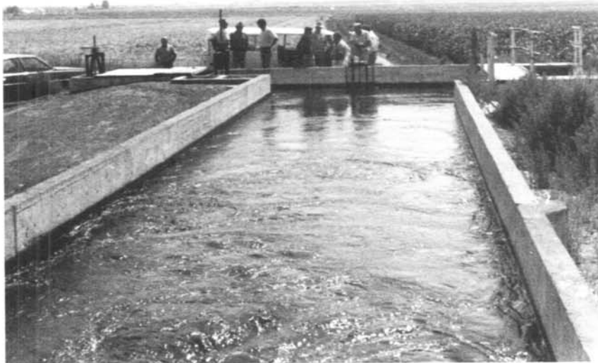
Figure 9. Square concrete stilling wells were constructed to replace round pipe stilling wells.
