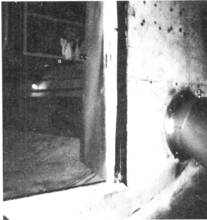
Figure 8.—Collapsed door to penstock tunnel.
