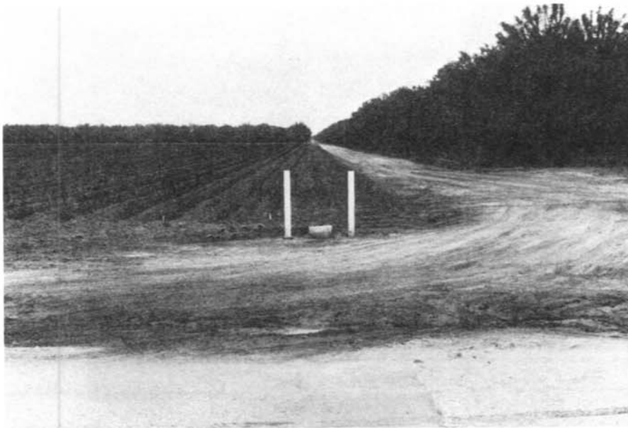
Figure 4.—Valve boxes extended above the ground and posts placed on the sides to prevent farmers from hitting them.
