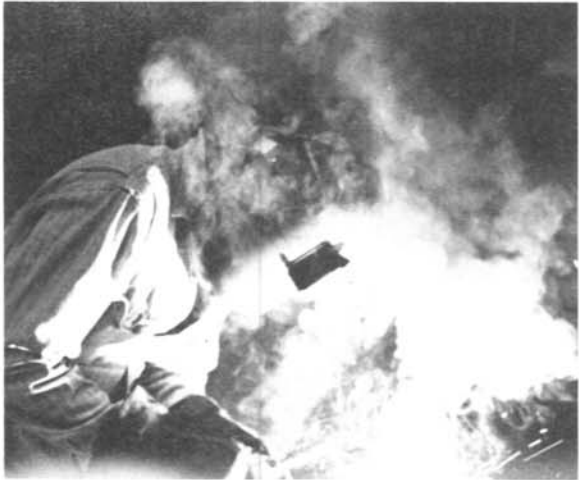
Figure 21.—Materials being welded may be coated with substances that produce toxic fumes during welding. Without proper ventilation, fumes can engulf a welder.
