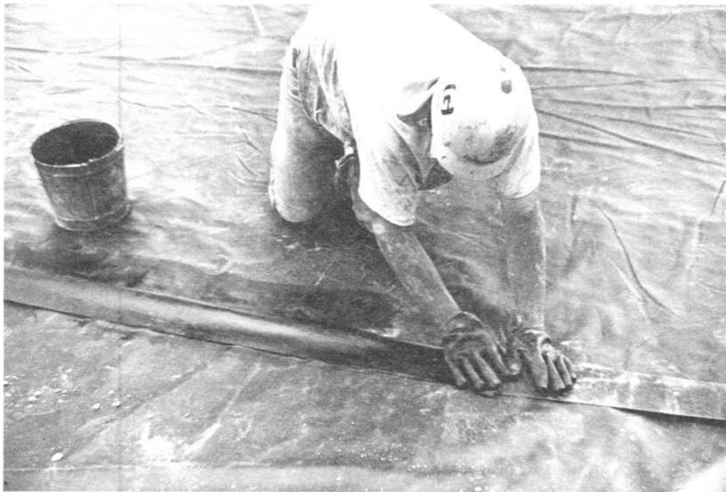
Figure 15.—Seams joining panels were sealed with special adhesive, then tested with an air gun. After inspection, a capping strip was applied.
