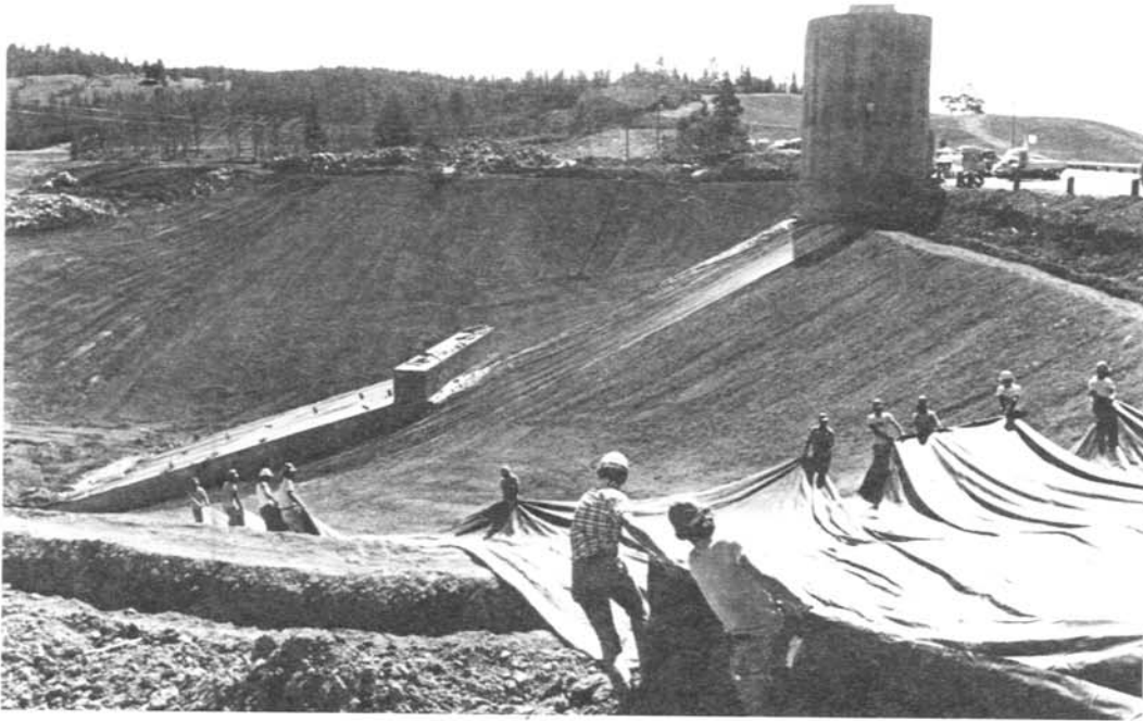
Figure 14.—Installation crew positions section of the membrane liner. Each section measures 1300 \text{ m}^2 (14 000 \text{ft}^2 ).
