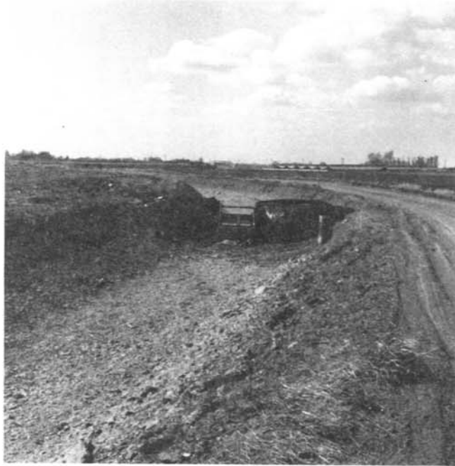
Figure 5.—Bulkhead/weir No. 2 with water stage recorder setup for inflow-outflow test on April 8, 1981.
