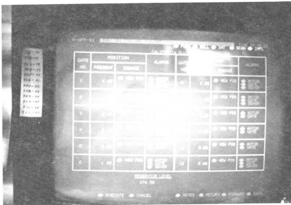
Figure 8.—CRT display at Imperial Diversion Dam control center.
