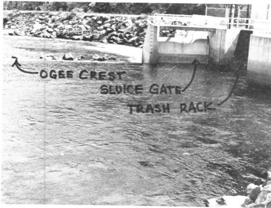
Figure 18—Sluice gate opening is maintained by the controller to hold a constant pool level.
