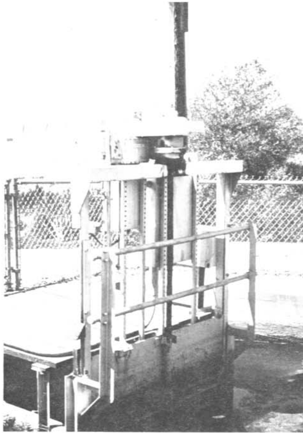
Figure 12.—Automated slide gate check structure.
