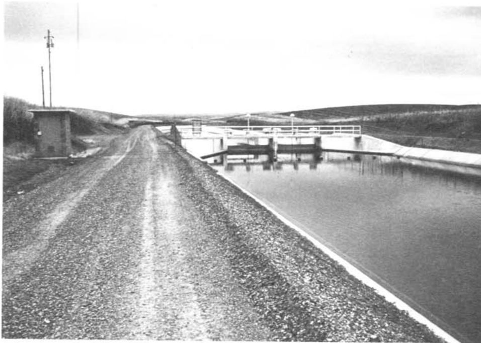
Figure 15.—Check structure. Control equipment shelter to left of road.
