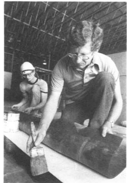
Figure 8.—Al Dedrick (foreground) and the BLM's Mark Nolte glue and lap the rubber sheeting together to form the stock pond covers.
