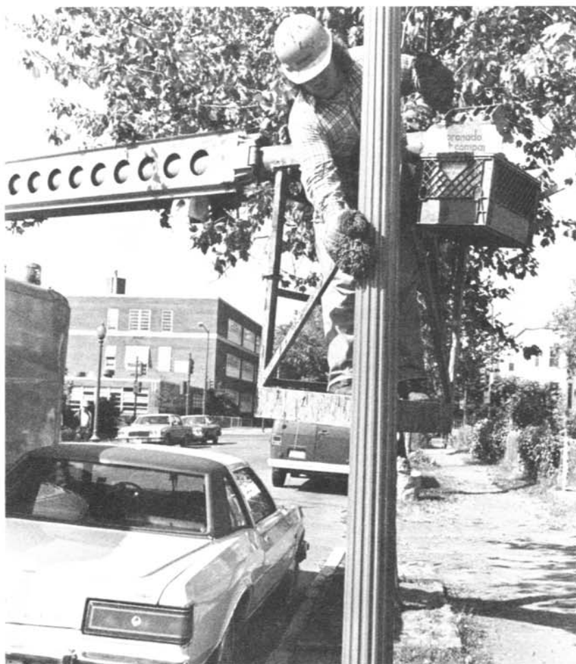
Figure 4.—Boom enables painter to paint any portion of the pole that cannot be reached from ground level.
