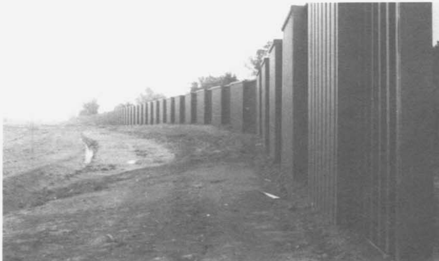
Figure 7.—Besides being easy to clean, the steel highway noise barrier will shield neighborhood from traffic noise.
