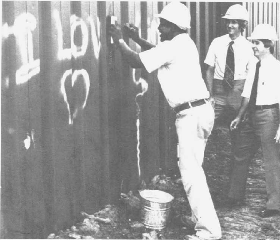
Figure 8.—Wall panels of steel highway noise barrier are covered with washable plastic film to permit easy graffiti removal.
