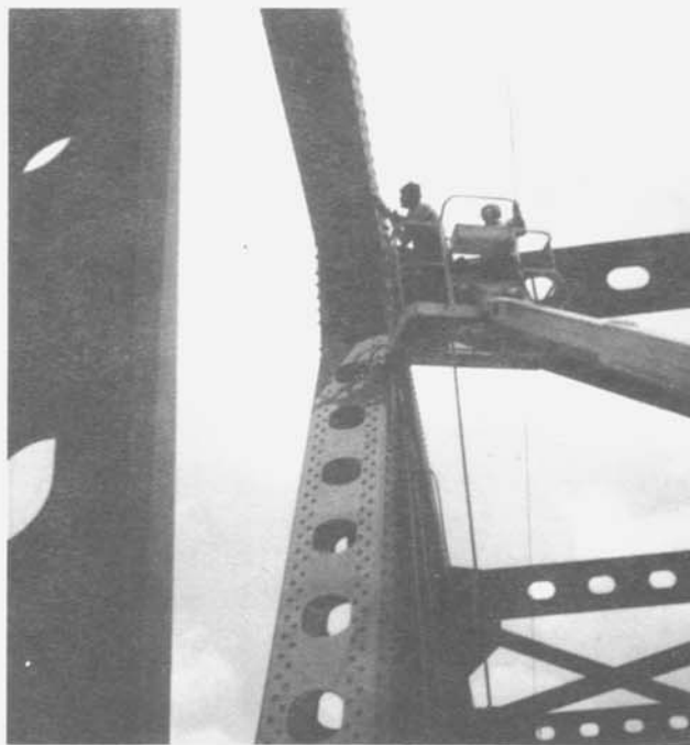
Figure 19. Workmen use 0.31-kg (11-oz) cartridges of caulk to seal voids in prime coat prior to completing bridge painting project.
