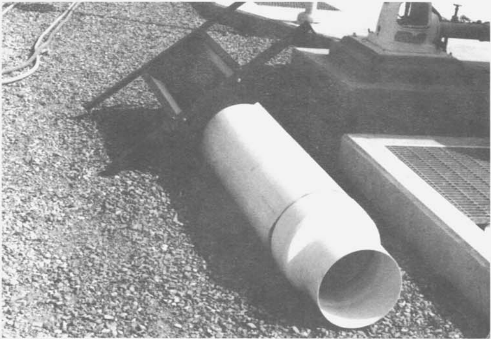
Figure 6. PVC pipe and opening for entry of wash water and moss.
