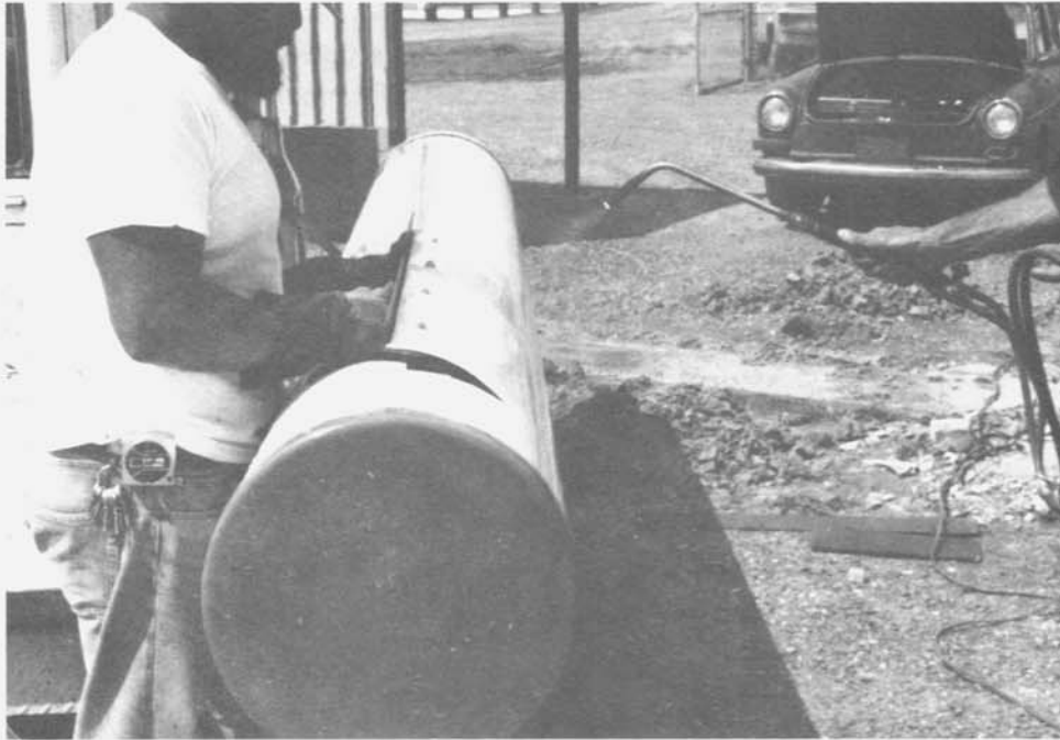
Figure 4. Applying heat to 380-mm (15-in) PVC pipe to allow forming a trough without cracking
