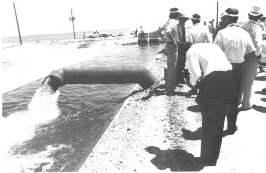
Figure 1. - The irrigation tailwater flow down this ditch is 631 \ell /s (10 000 gal/min). The solar powered irrigation pump located 4.27 m (14 ft) away delivers water from a tailwater pond to the ditch.
